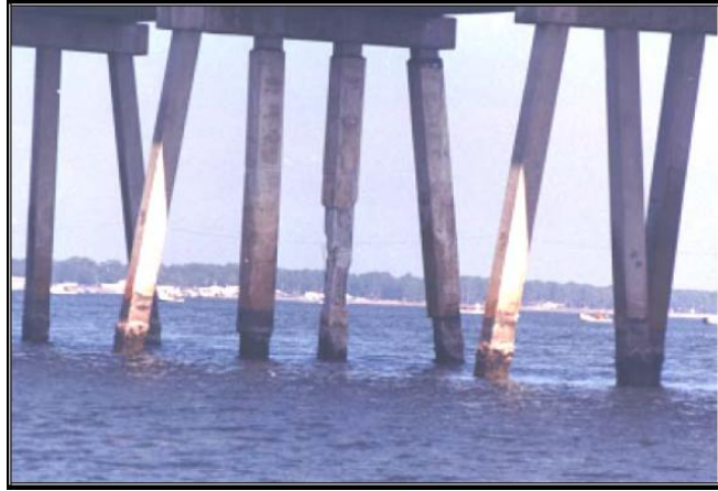
Figure 1-3 Bryant Patton Bridges displaying reinforced concrete piles with significant corrosion induced damage-Florida. (D.V.Reddy,2006)
