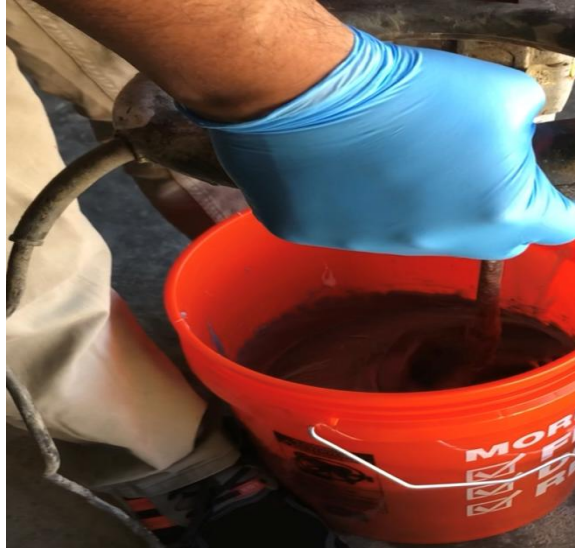
Figure 3-5 Epoxy resin (Parts A and B) were mixed using an electric paddle.
