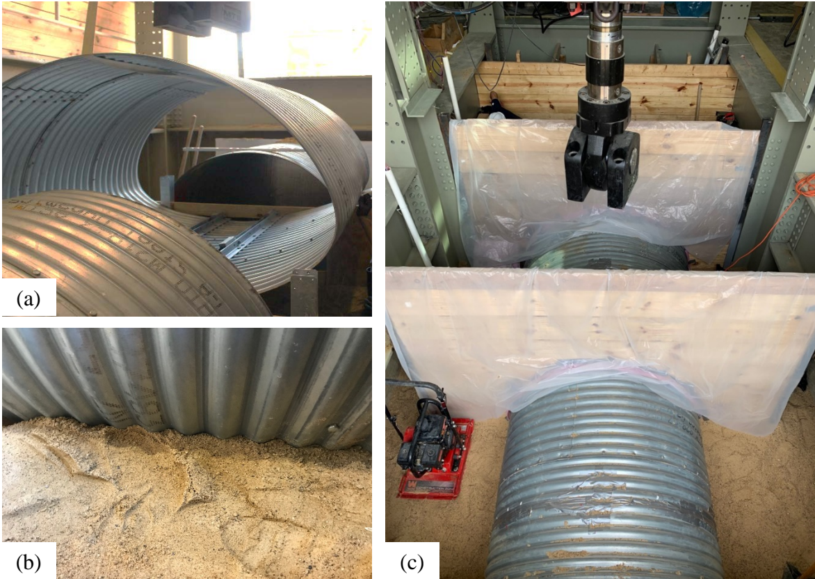
Figure 3-25. Test setup configuration for all three cells: (a) during CMP installation, (b) during embedment, and (c) filled hunch area with poorly graded sand without compaction.
