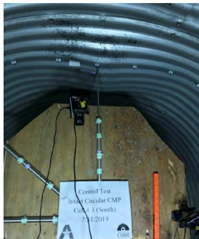
Figure 4-1. Intact CMP with local buckling at the crown location.
