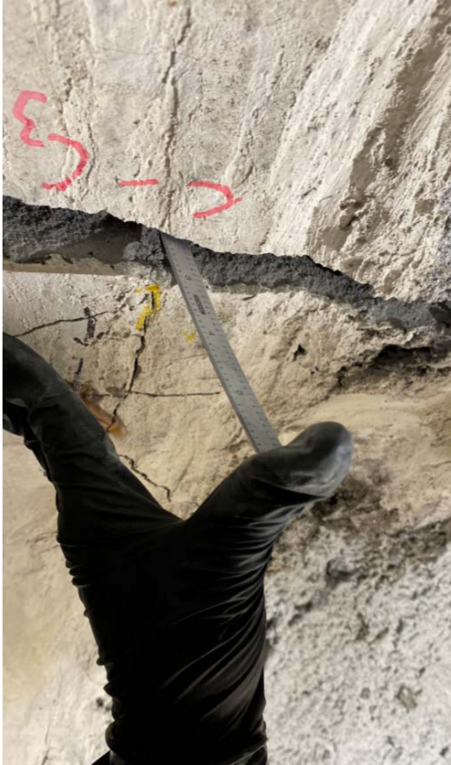
Figure G-29. Crack opening at the crown location of the 3-in. thick circular SAPL renewed CMP at the end of the test.
