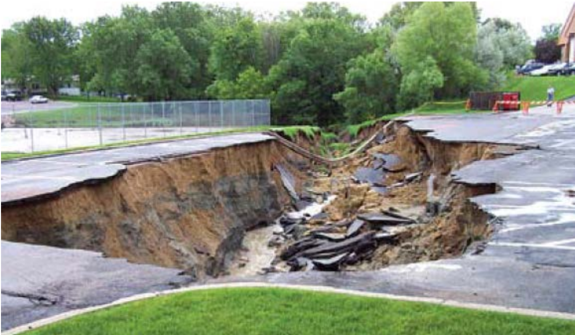
Figure 1-3. Culvert failure in South Dakota (ACPA 2008).
