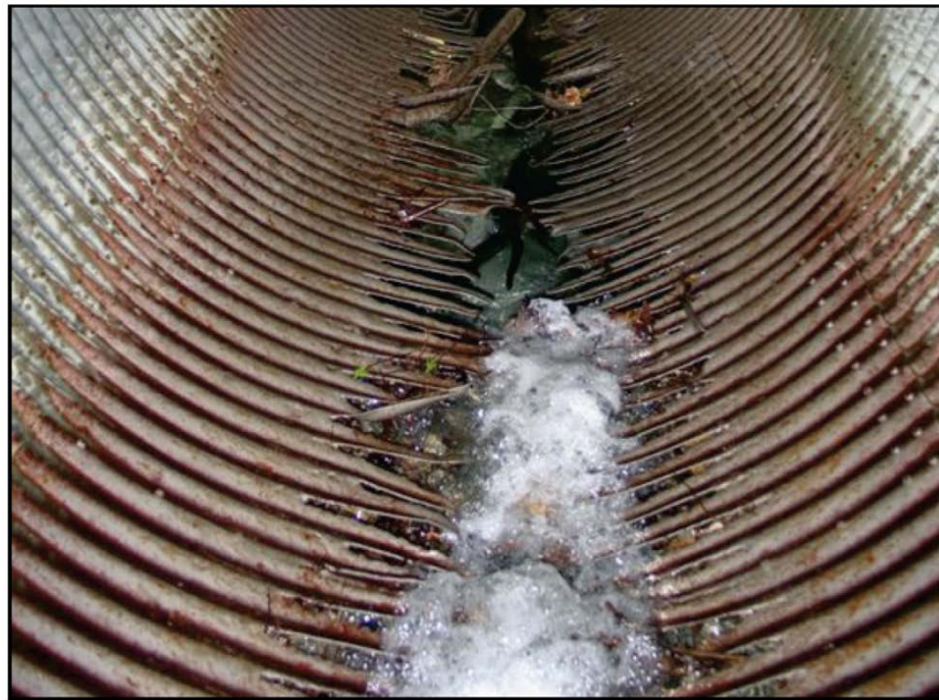
Figure 1-12. Fully invert deteriorated CMP culvert (FHWA 2012).
