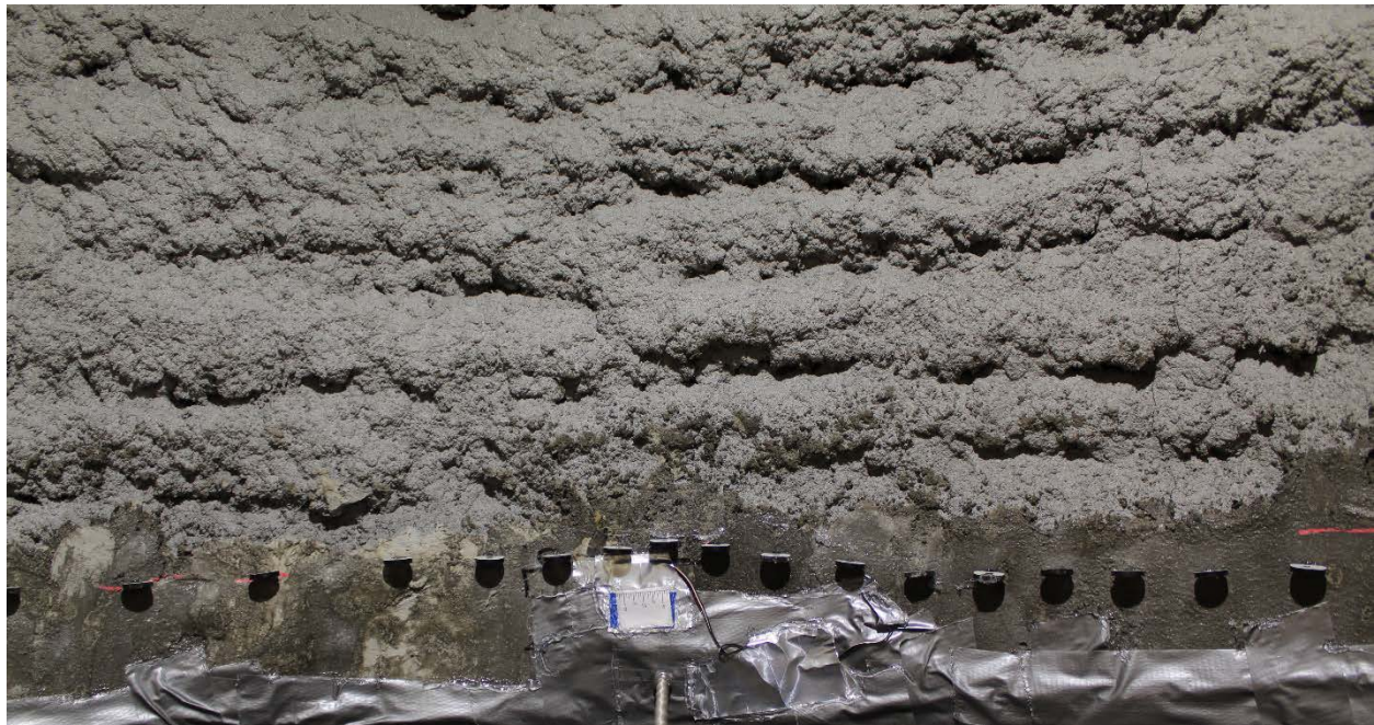
Figure F-9. Crack width measurement on the crown of the 2 in. SAPL renewed circular CMP at the beginning of the test.
