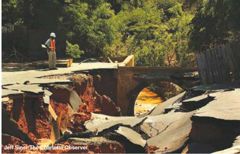
Figure 1-4. A 96 in. culvert failure in Hickory, North Carolina (ACPA 2008).
