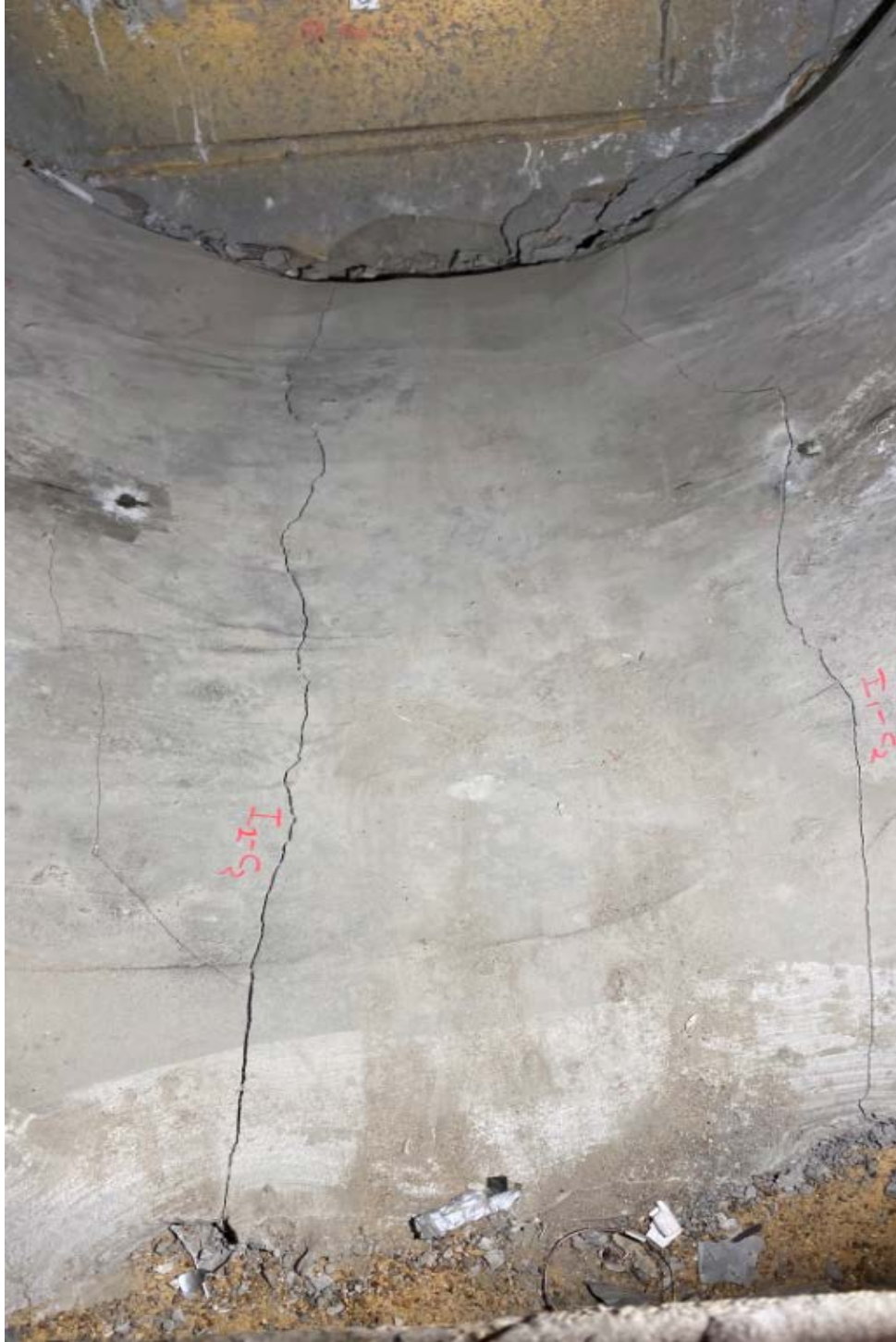
Figure G-30. Longitudinal cracks at the both gaps of the invert-cut section.
