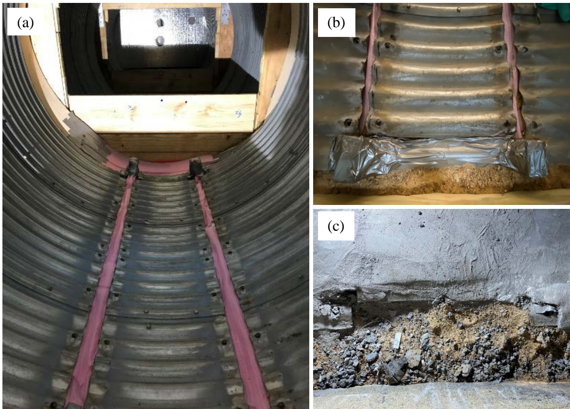
Figure 3-36. End-strip detachment: (a) end-strip preparation, (b) end-strip before SAPL installation, end-strip detachment after SAPL installation.
