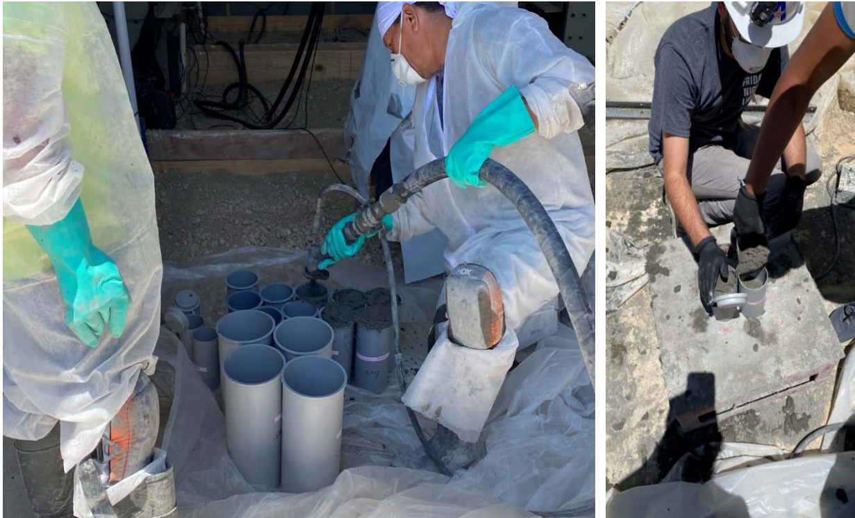
Figure 3-44. SAPL casting method into the cylinders: (left) spray-cast, and (right) hand-cast method.
