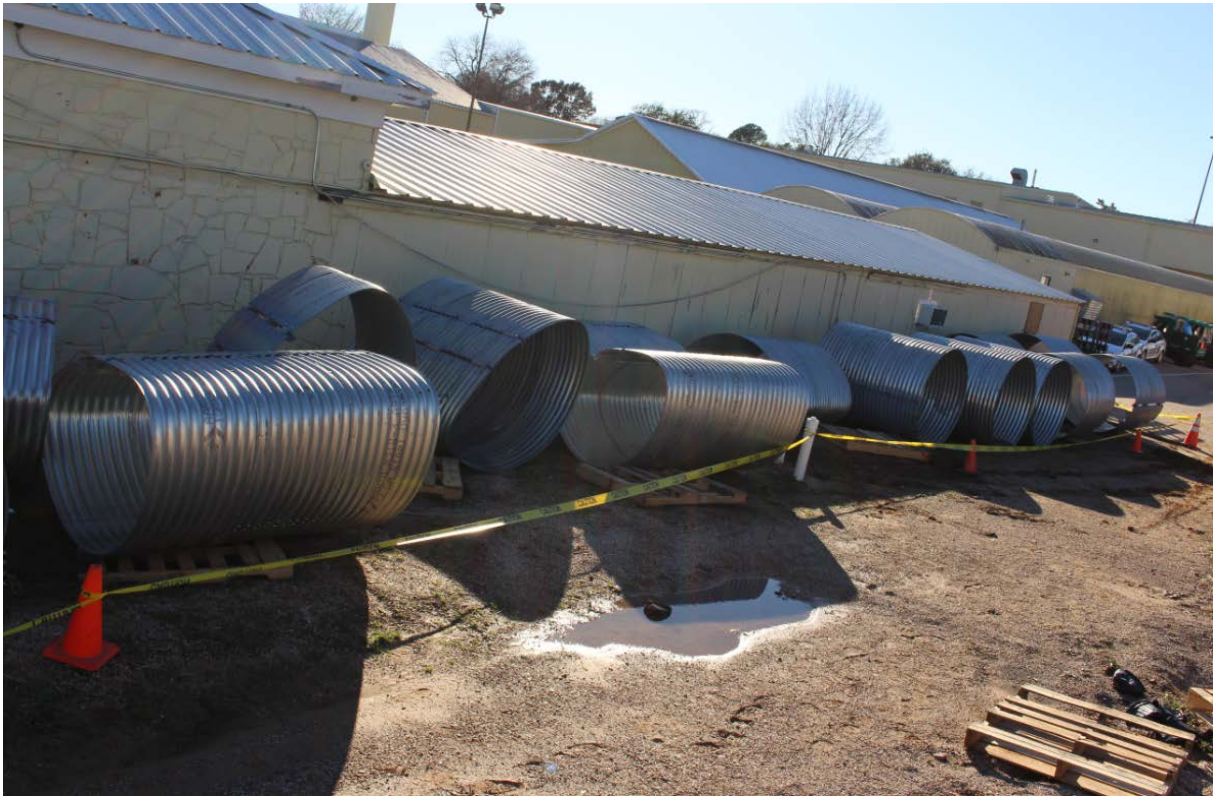
Figure G-2. CMP unloading and storage
