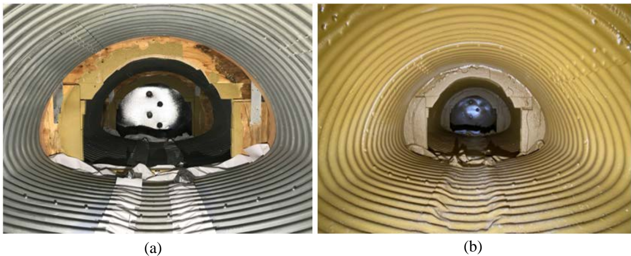
Figure 1-26. Hand spray polyurethane SAPL: (a) before renewal, and (b) after renewal (Kohankar Kouchesfehni 2020).
