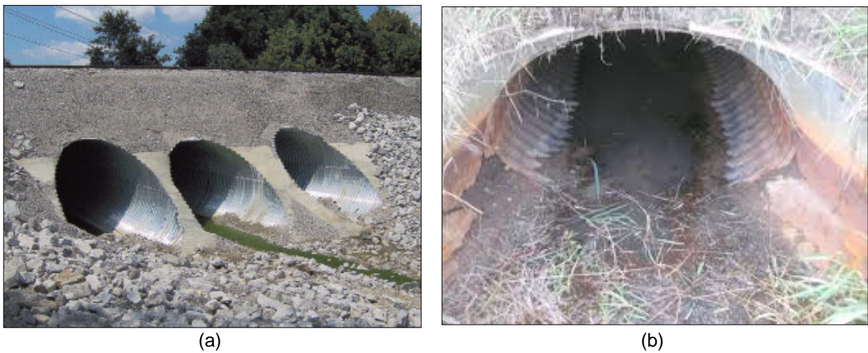
Figure 1-2 Corrugated metal pipe culverts (CMPs): (a) multi-cell CMPs (Source: Contech), and (b) invert deteriorated CMP (Source: Metal Culverts Inc.).
