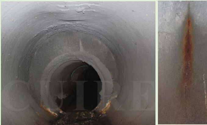
SAPL Irregularities at the Crown, Iron Oxidation on SAPL Surface below the Springline
