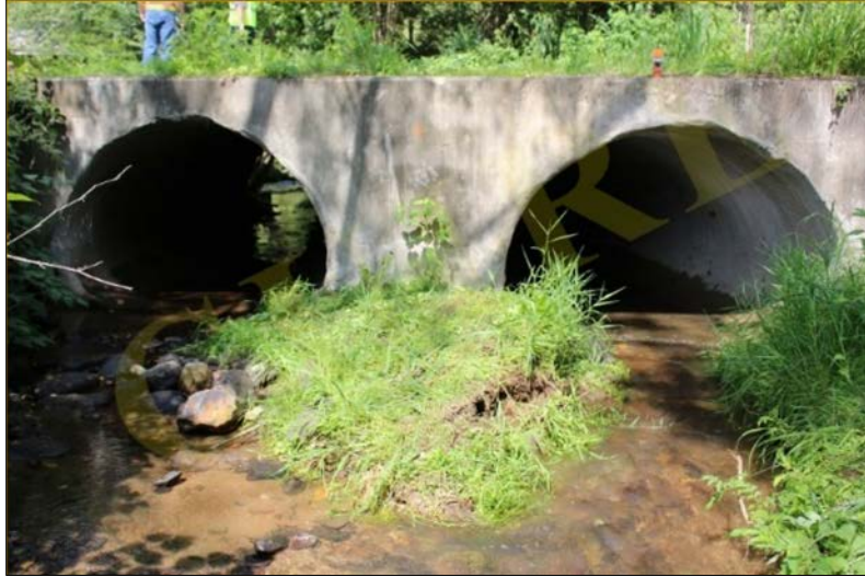
Figure 1-24 A sample of SAPL renewed twin culvert, North Carolina (Photo by Zahra Kohankar Kouchesfehni, CUIRE).
