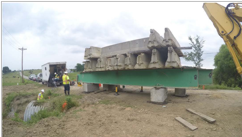
Figure 2-8 Field testing of a shallow cover severely deteriorated arch CMP (Sargand et al. 2018).
