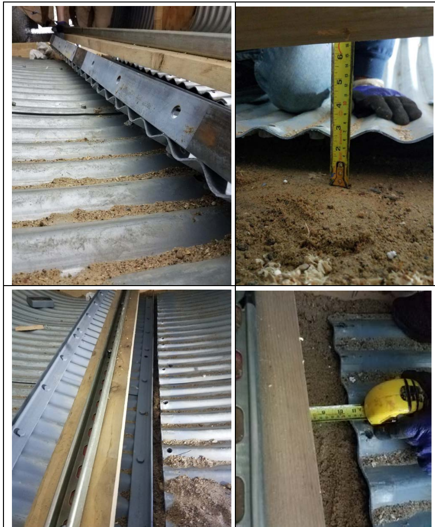
Figure 5-1 CMP movement due to the invert detachment (without any end strips) before loading.
