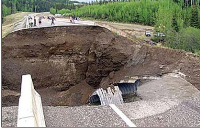
Figure 1-17 Culvert failure in British Columbia, Canada (American Concrete Pipe Association 2008).
