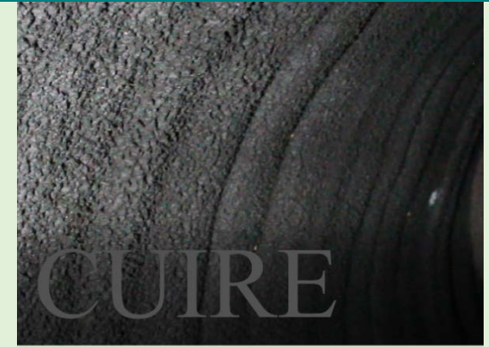
Inconsistent SAPL Thickness On RCP
