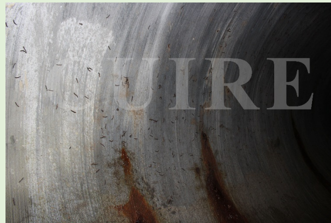
Worms on the Liner Surface (Vermin)
