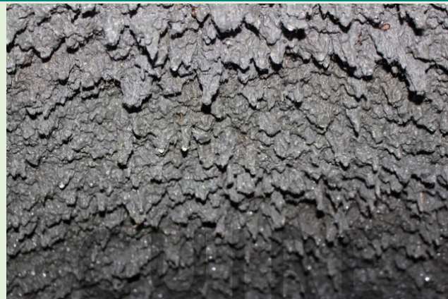
Heavy and Rough Material at the Crown
