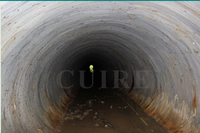
Corrosion of Metal pipe with Iron Oxidation on Liner Surface, Aggregate Deposits at Invert
