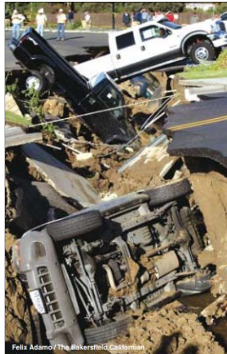
Figure 1-18 Culvert failure in Bakersfield, California (American Concrete Pipe Association 2008).
