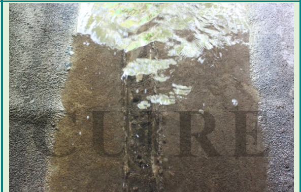
Invert Problem (Installation Problem)
