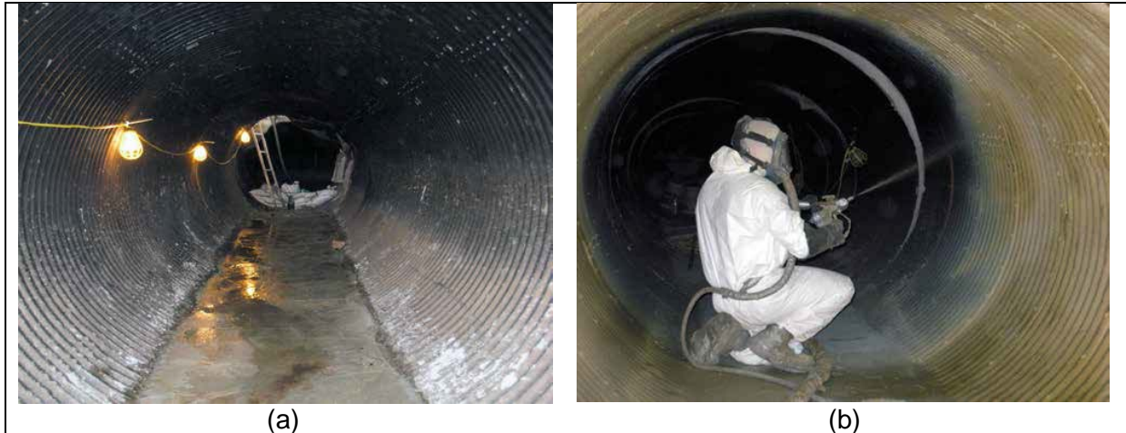
Figure 2-2 CMP renewal using SprayWall® Polyurethane SAPL, Norristown, PA: (a) Before Renewal, and (b) CMP Renewal during SAPL Application, 2007 (Sprayroq Inc.).
