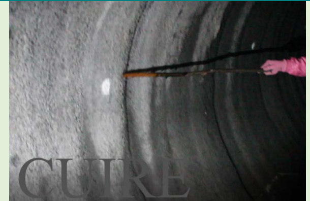
Inconsistent SAPL Thickness both Sides of RCP Joint
