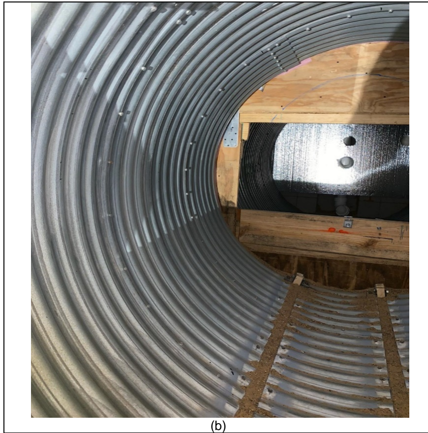
Figure 4-14 CMP surface preparation for SAPL installation: (a) dirt and dust on the CMP, and (b) CMP after power wash without any dirt and dust.
