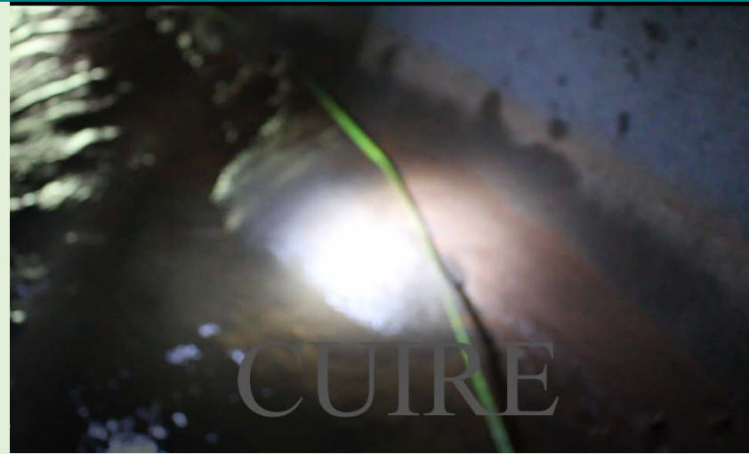
Settled Deposits (Hard/Compacted)
