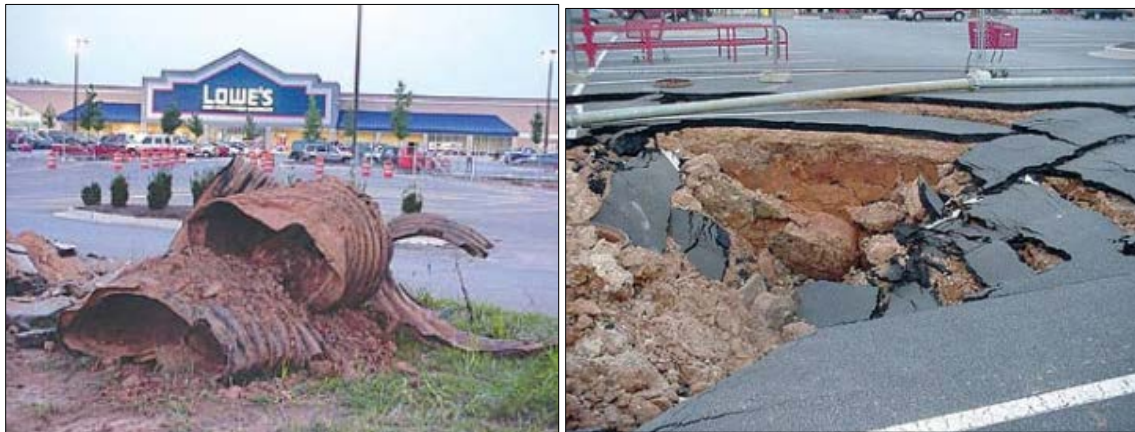
Figure 1-16 Culvert failure in Timonium (American Concrete Pipe Association 2008).
