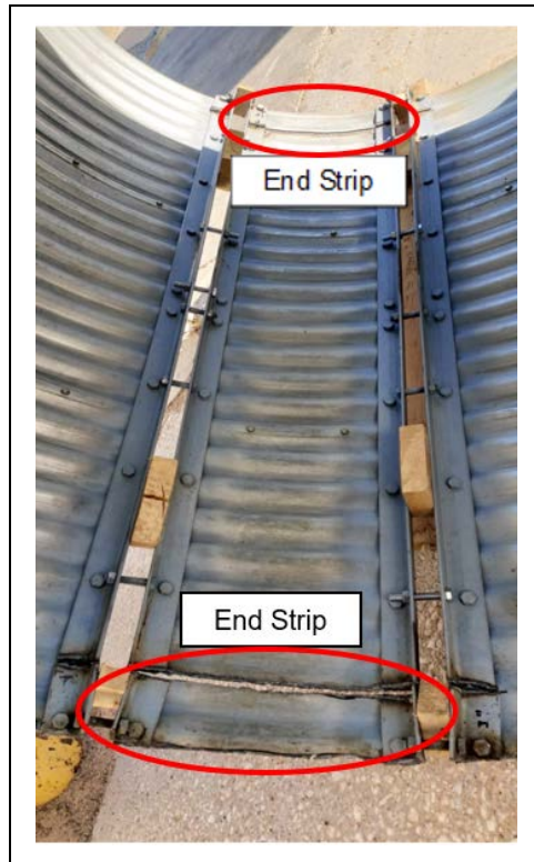
Figure 4-6 End strips of the invert-cut CMP samples.
