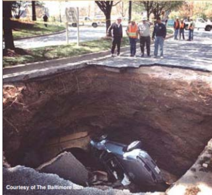
Figure 1-15 Culvert failure in Maryland (American Concrete Pipe Association 2008).
