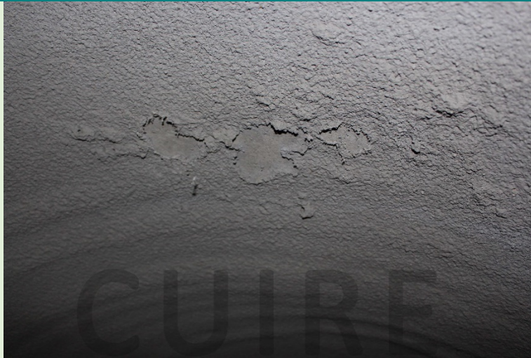
Delamination at the Crown
