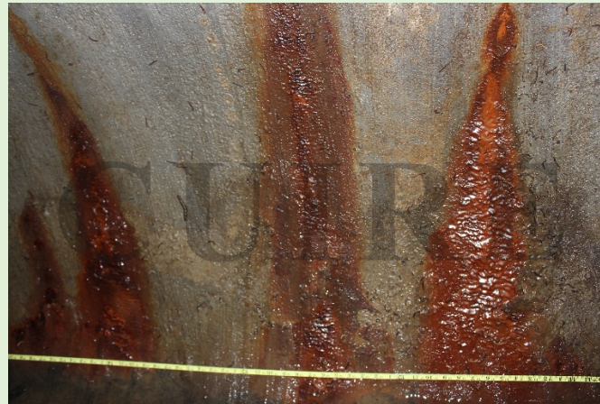
Corrosion of Metal pipe with Iron Oxidation on Liner Surface
