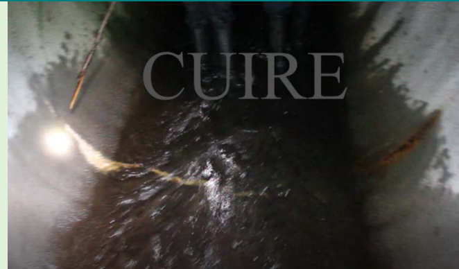
Circumferential Crack through the Invert Iron Oxidation, Efflorescence
