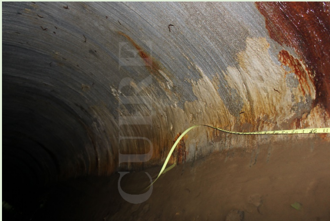
Inconsistent Thickness Concrete Patching on the Liner Surface
