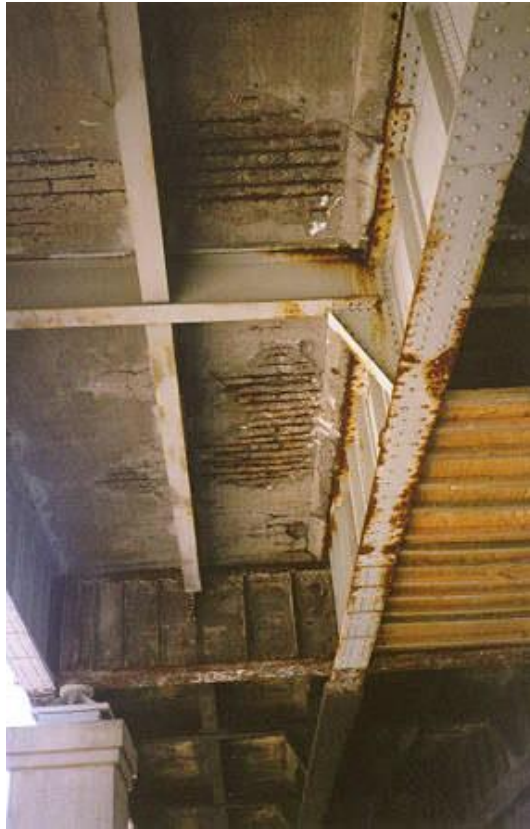
Figure 1-1 Significant bottom delamination
