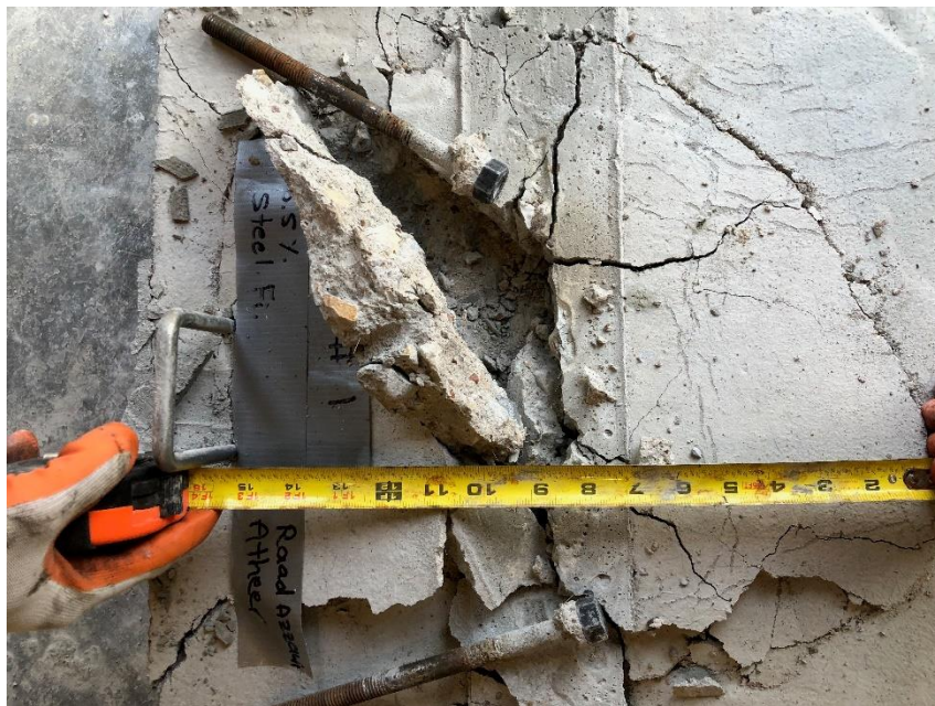
Figure 3.25 Concrete Breakout Failure (0.5% SFRC)
