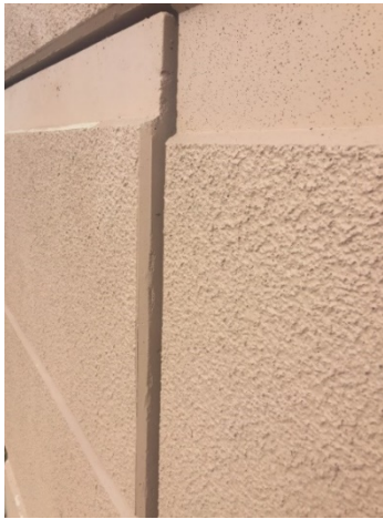
(a) Differential movement between panels at Walls CC1-3
