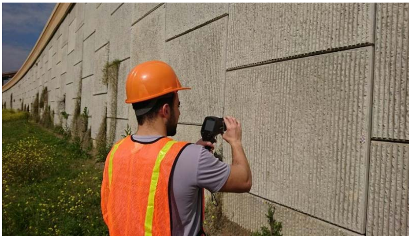
Figure 4-19 Infrared camera scan at Wall 264R
