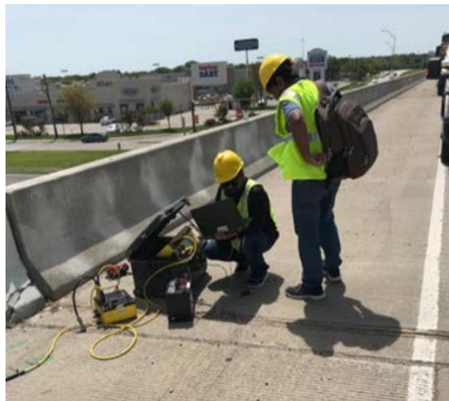
(d) Connecting the RI cable to Multi Electrode Switch Box and RI SuperString, and conducting RI scan
