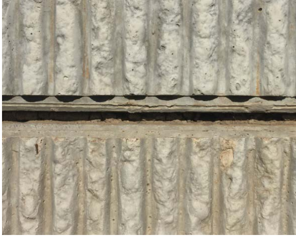
(a) Backfill leakage and wide joint opening at Wall 264R
