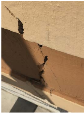
(a) Cracks on wall coping at Wall 179L
