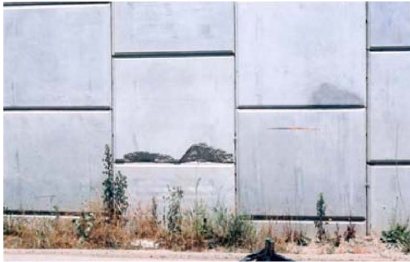
Figure 1-4 Spalling of concrete near failed bearing pads (Neely and Tan 2010)
