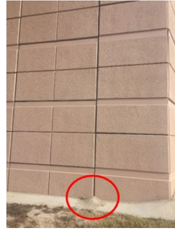
(c) Leakage of backfill soil at Walls CC1-3
