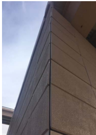
(b) Opening of corner joint at Walls CC1-3
