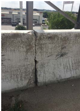
(b) Cracks on traffic barriers at Wall 179L
