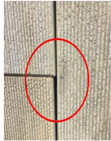
(c) Differential movement between panels at Wall 179L
