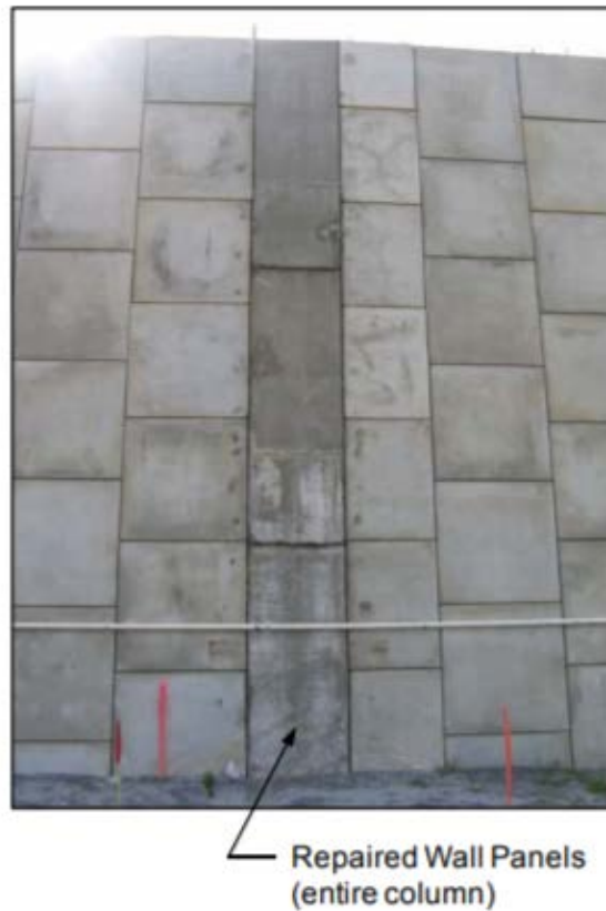
Figure 2-1 MSE wall repair (Kim et al. 2010)
