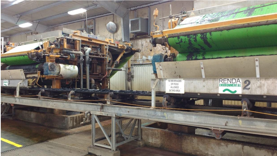
Figure 3.19: Biosolids from the sludge dewatering facility
