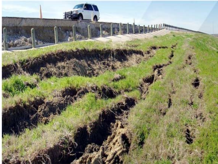
Figure 3.12 Typical slope failures occurred (a) Grapevine and (b) Joe Pool dam (Courtesy: USACE, Fort Worth District; Dronamraju 2008)
