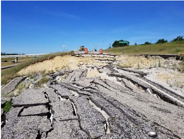
Figure 6.2 Failed portion of slope
