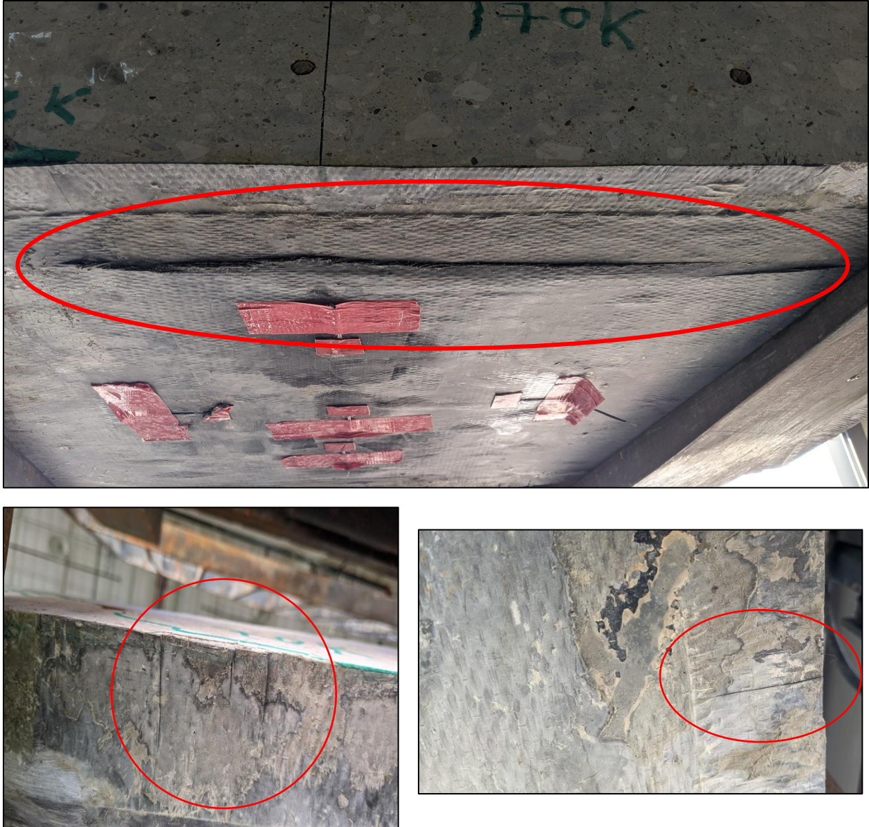
Fig 5.10: Rupture of transverse CFRP fabric
