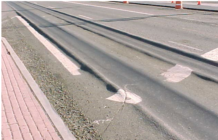
Figure 2.2 Severe mix rutting [15]
