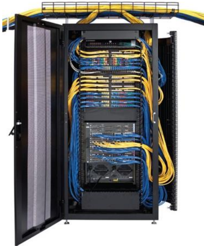
Figure 4- 7. Cables inside cabinet [13]
