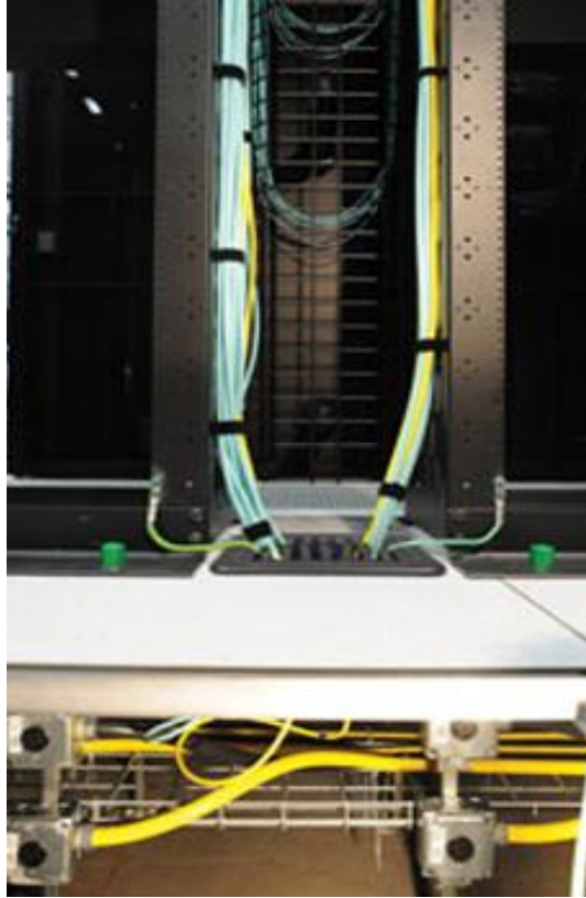
Figure 4- 4. Cabinet cable penetration seal
