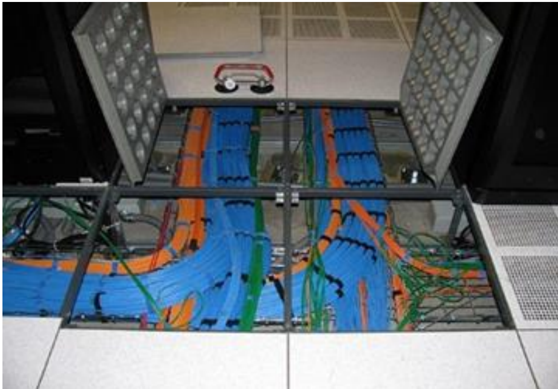
Figure 4- 3. Underfloor data cables [11]
