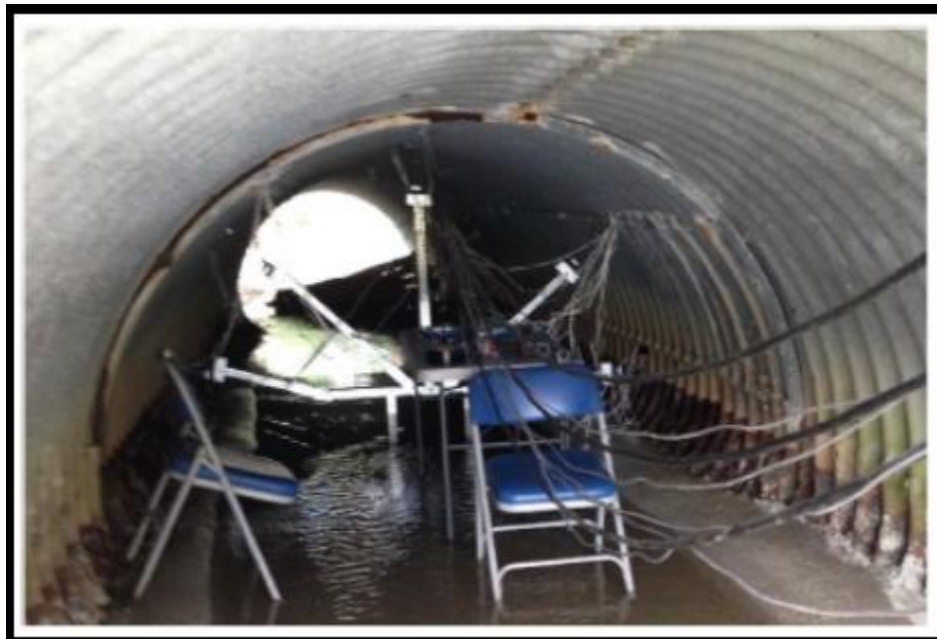
Figure 2-13 (a) Load Configuration for testing (b) Invert Deteriorated Pipe with instrumentation (Sargand, Khoury, & Hussein, 2018)
