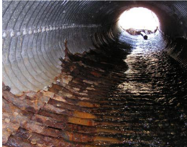
Figure 1-2 Deteriorated Metal Culverts (Taher & Moore, 2011)
