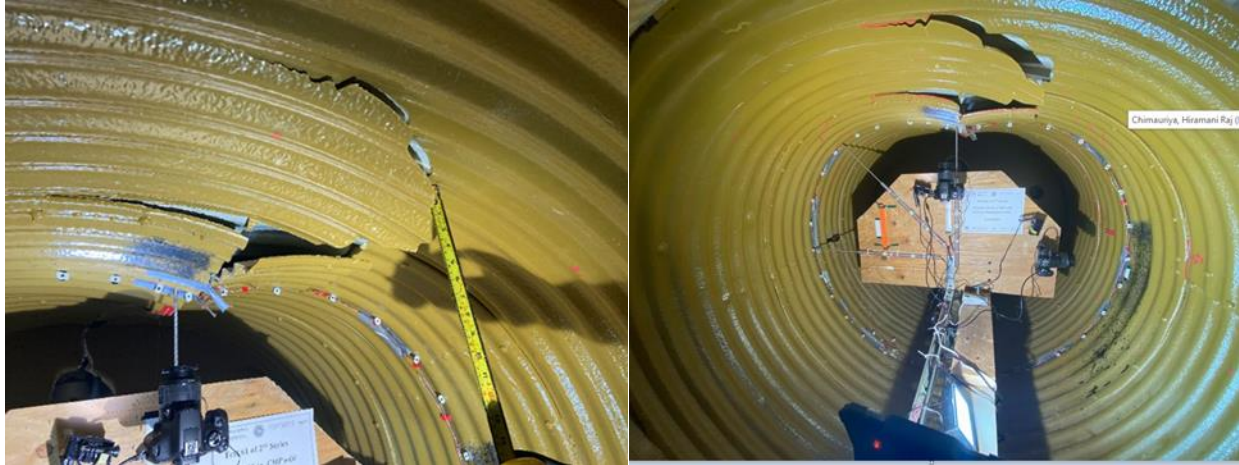
Figure 3-57 Cracks in lined CMP after the completion of test for 0.25 in. thick liner (Source: CUIRE Laboratory)
