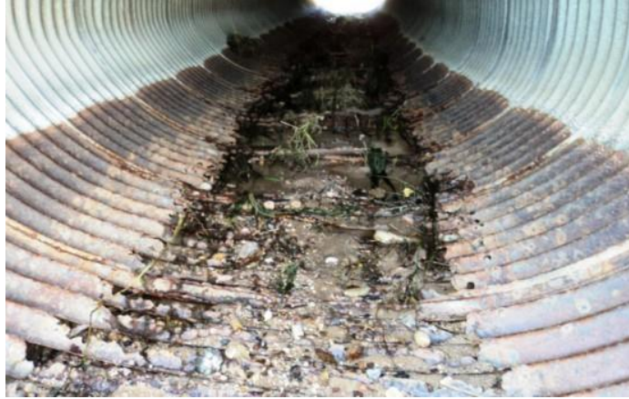
Figure 2-8 CMP with complete loss of invert (Colorado DOT, 2014)
