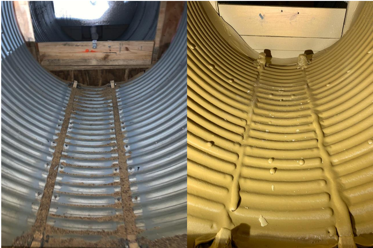
Figure 3-54 Invert detached CMP before and after the application of the liner (Source: CUIRE LAB)
