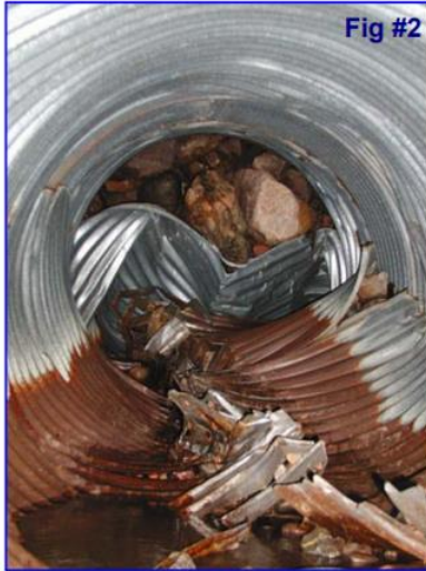
Figure 2-10 Failure of CMP due to buckling (Tenbusch & Dorwart, 2009)
