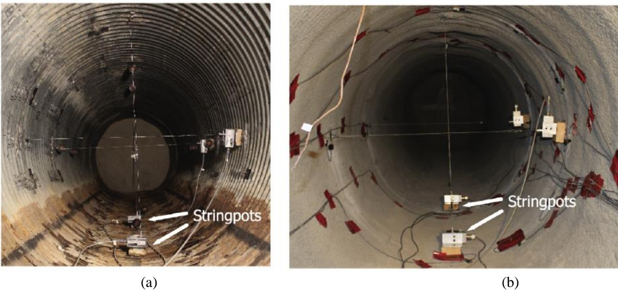
Figure 2-17 (a) Pipe before the application of the liner (b) Pipe after the application of the liner (Garcia & Moore, 2015)
