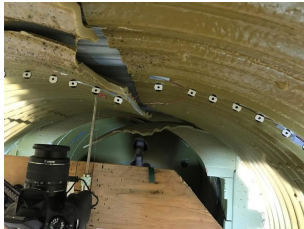
Figure 3-63 Crack in 0.5 in. thick liner after the completion of test for 0.5 in. thick liner (Source: CUIRE Laboratory)
