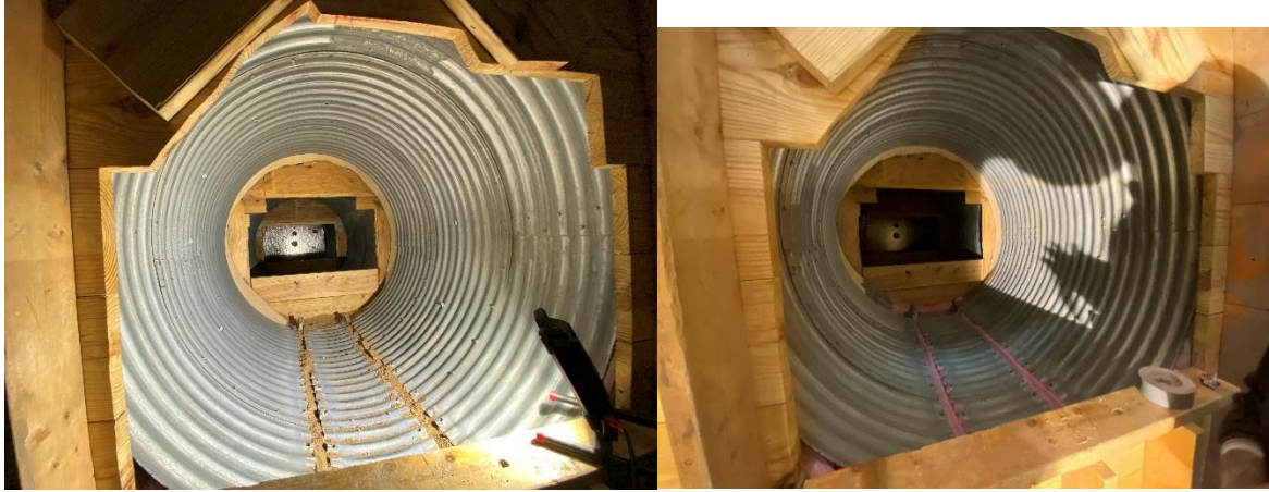
Figure 3-36 (Left) CMP just after removal of the invert (b) CMP ready for lining (Source: CUIRE LAB)
