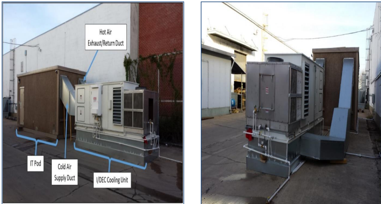
Figure – 7: Data center at Mestex Dallas facility [12]
