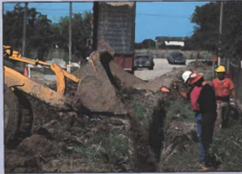
A construction crew places a section of water pipeline in Cameron Park. The $5.2 million project will be complete by October 1994.
