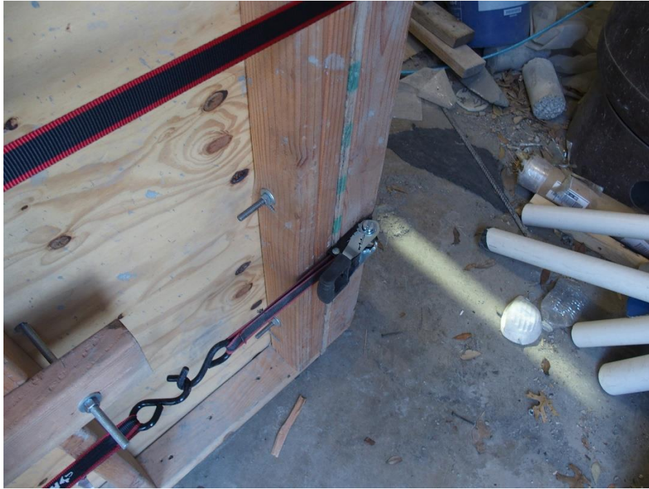
Figure 4-79 Rope used as extra safety to prevent the supporting block to open during concrete casting
