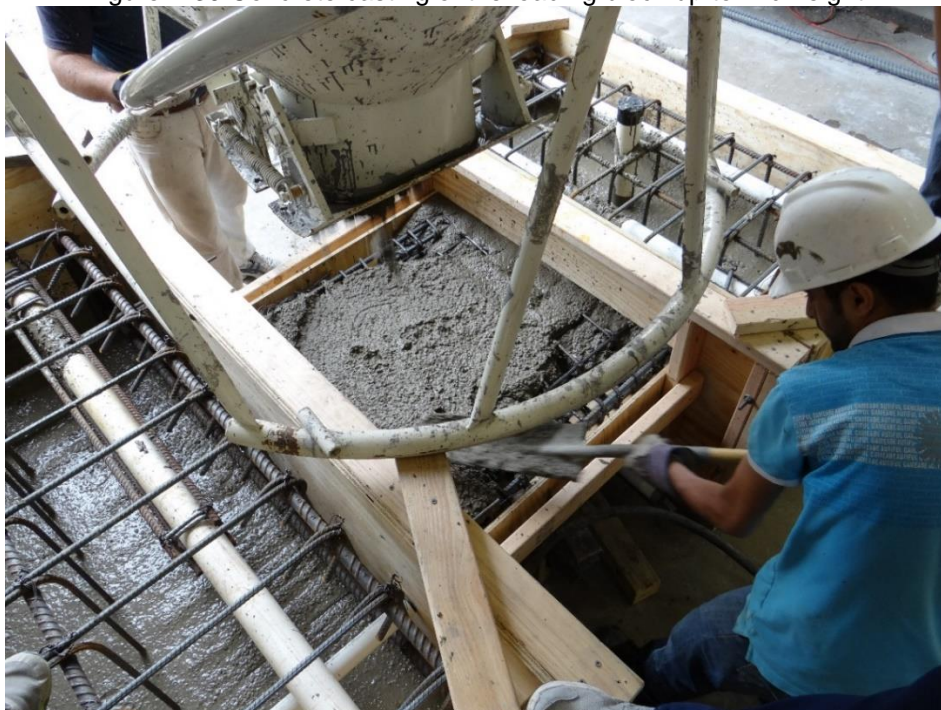
Figure 4-40 Concrete casting of the supporting and loading blocks up to mid height and wall casting.
