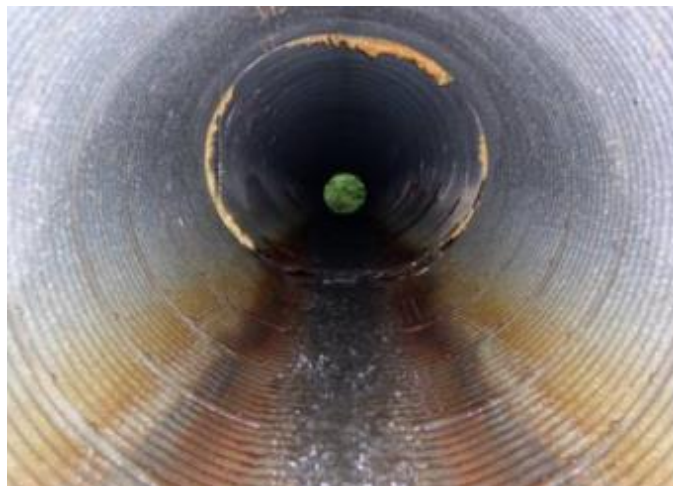
Figure 1.4. An Invert Corroded CMP Culvert Source: cuire.org
