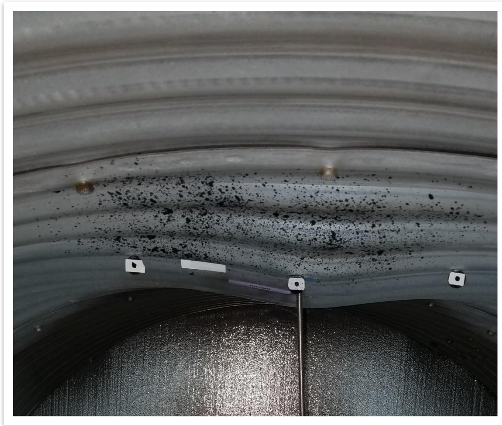
Figure 6.8 Bare CMP Deflection
