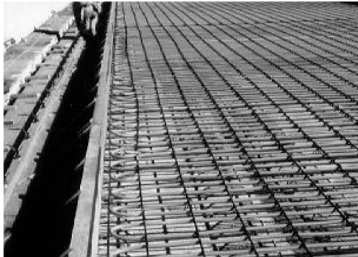
Figure 2-20. Heating hoses in place ready for concrete pour; hoses are on 152 mm (6-in.) centers placed 76 mm (3 in) under the top of the slab, affixed below #4 rebar
