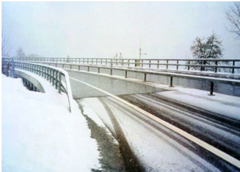
Figure 2-19. SERSO system in operation (Eugster, 2007)
