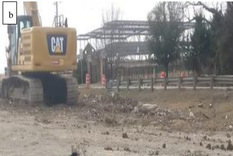
Figure 21 Site clearing works (a) Approximate site clearing area (b) Ongoing site clearing works
