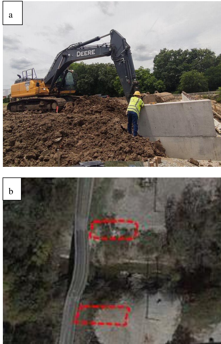
Figure 25 Backfilling works (a) Backfilling works boundary, (b) Ongoing backfilling works at site
