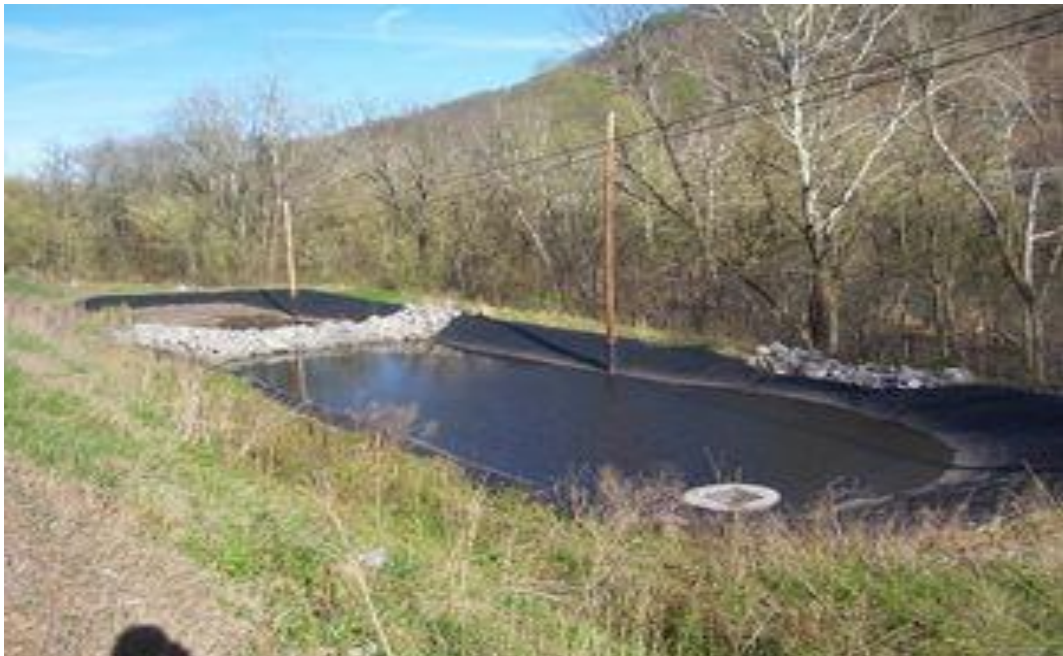
Figure 9 Sediment retention pond (TxDOT 1993)
