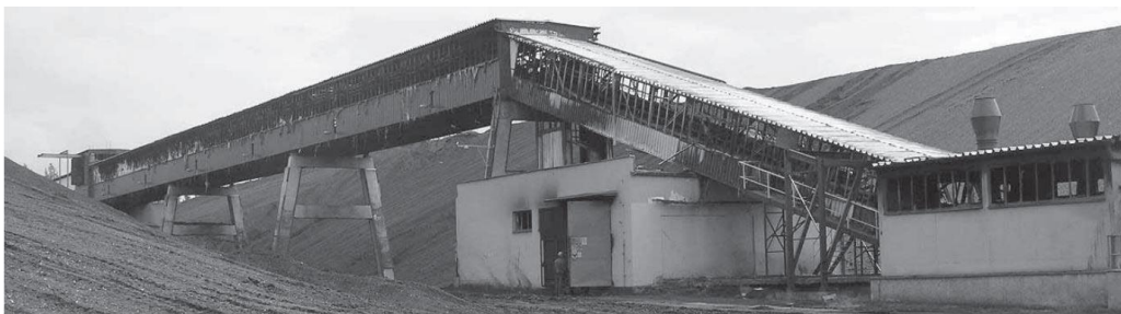
Figure 2- 1: Fire-affected steel truss coal bridge evaluated based on tensile strength of structural steel (Wang et al., 2010).
