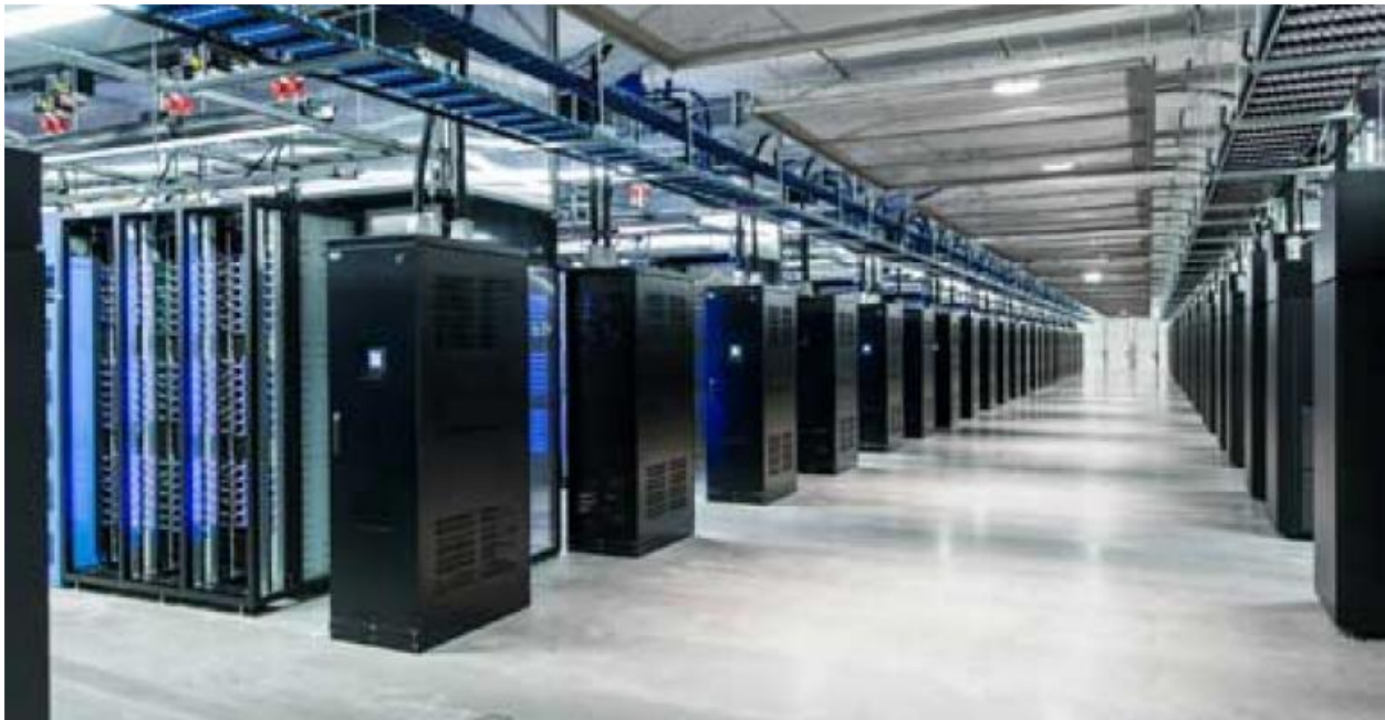
Figure 2 Facebook Data center [4]
