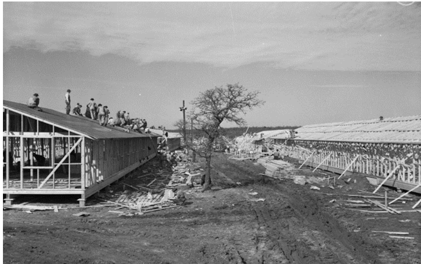
Figure 10: “Camp Wolters, Texas.” This photo shows laborers (left) laying tar paper for the roof of one of the numerous buildings during the construction of Camp Wolters. With camps going up across the country, building supplies became scarce, which delayed work on several occasions, Fort Worth Star-Telegram Collection , January 2, 1941, University of Texas at Arlington Libraries.
