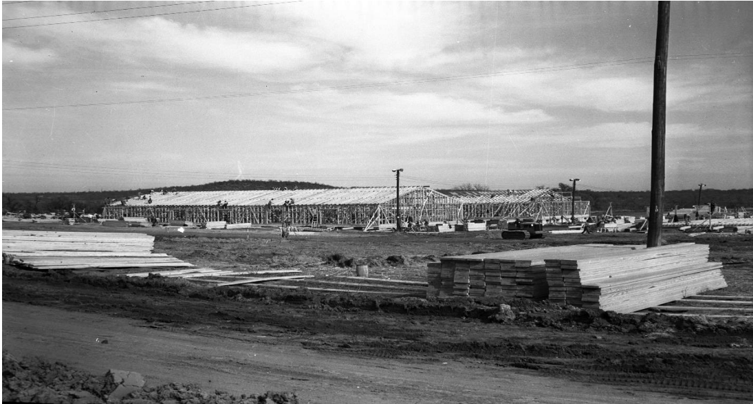
Figure 15: Construction workers framing buildings at Camp Wolters. Framework is completed on two buildings, while stacks of lumber lay in the foreground waiting to be used, Fort Worth Star-Telegram Collection, December 1940, University of Texas at Arlington Libraries.
