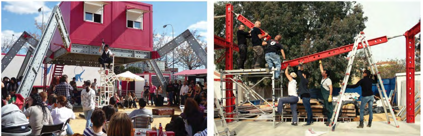
Figure 4.8 La Carpa Circus show, and during construction, 2014. Image courtesy Santiago Cirugeda, Resetas Urbanas.
