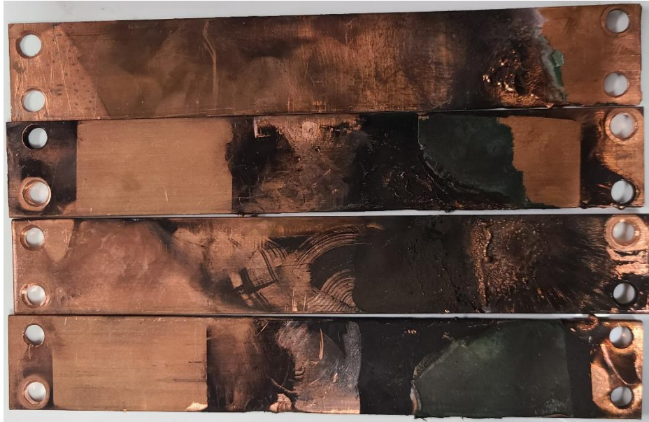
Figure 23 – Copper rails damaged by breakdown
