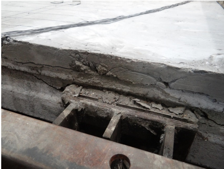
Figure 4-112 Local damage at the location of applied load.
