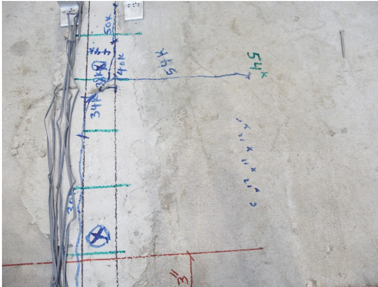
Figure 4-7 Starting the crack in the plank (fixed side) at 54 Kips.
