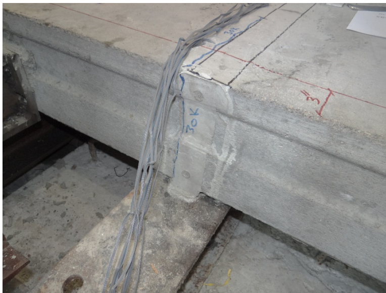
Figure 4-1 The first crack in the connection (at 30 Kips).
