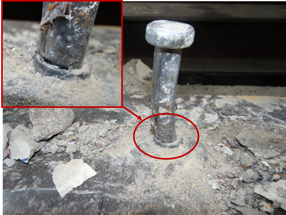
Figure 4-43 Fracture on the top of welding area of a stud at (+57 Kips).
