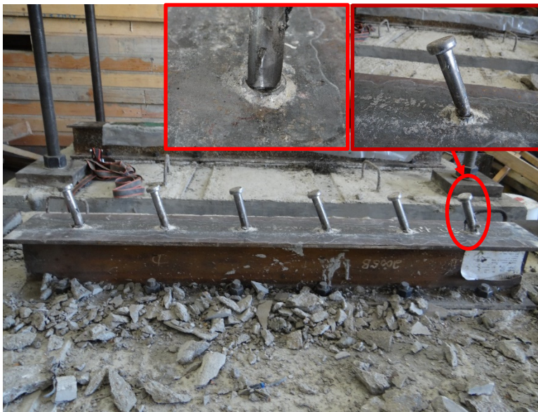
Figure 4-157 Yielding and fracture of shear studs.
