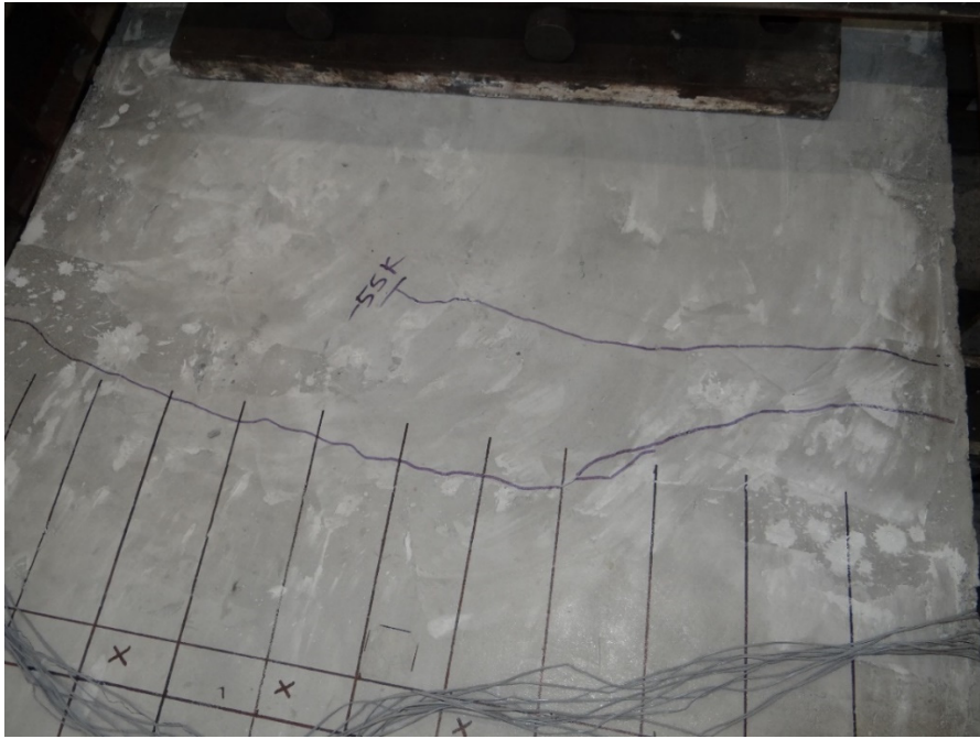
Figure 4-115 Cracks on the top of topping slab at (-55 Kips).
