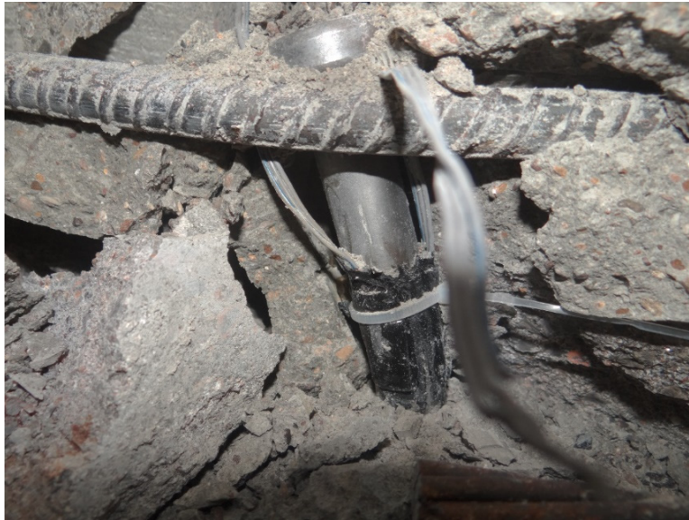
Figure 4-19 First Shear stud in the west direction, it started yielding at 49 kips.
