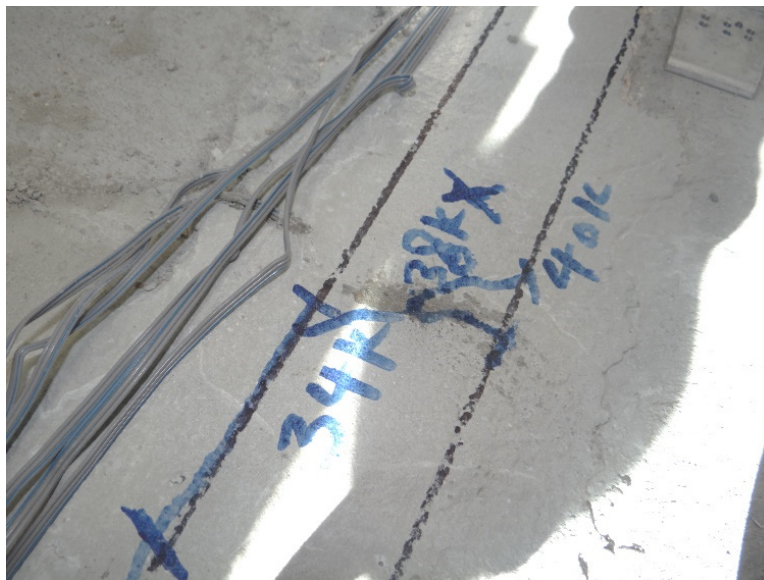
Figure 4-4 the second diagonal crack in the grout of the connection at 40 Kips.
