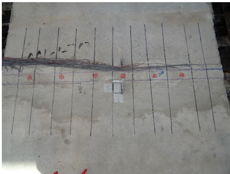
Figure 4-72 A new crack occurred in the roller side –west end at -30 Kips
