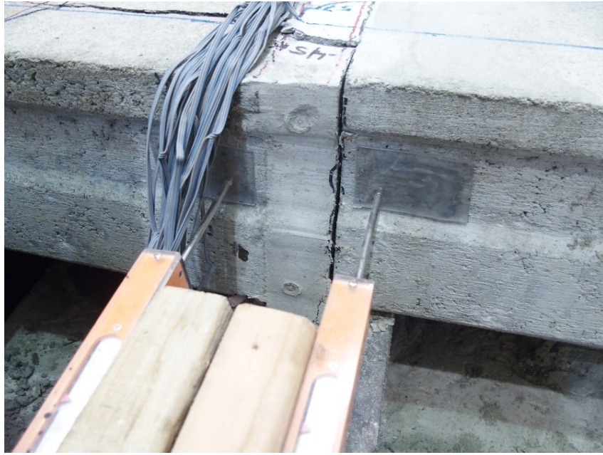
Figure 4-41 Failure in the ends of connection at (+57 Kips)
