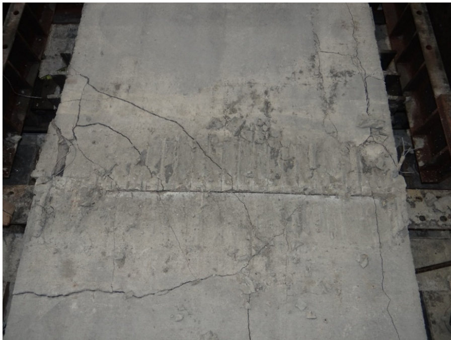
Figure 4-116 Cracks in the planks after removing topping slab.
