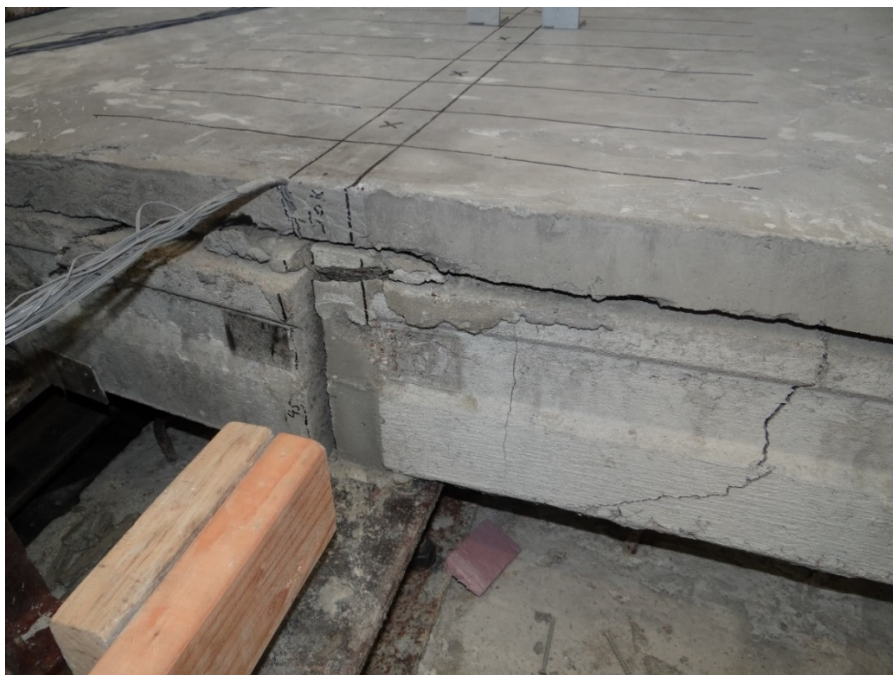
Figure 4-114 Failure in the ends of connection at (-55 Kips).
