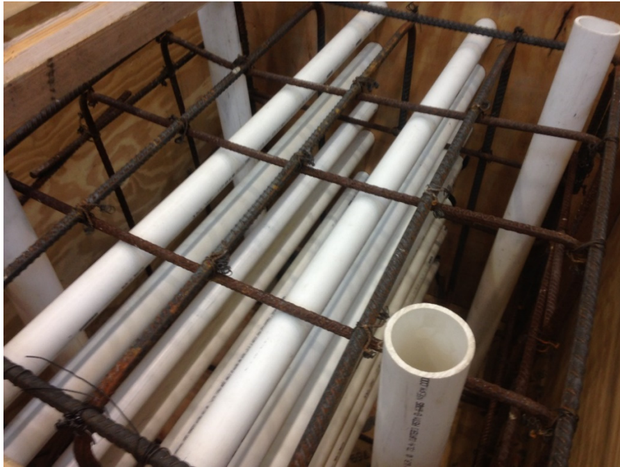
Figure 3-14 Horizontal and vertical PVC pipes to support the blocks and the actuator.
