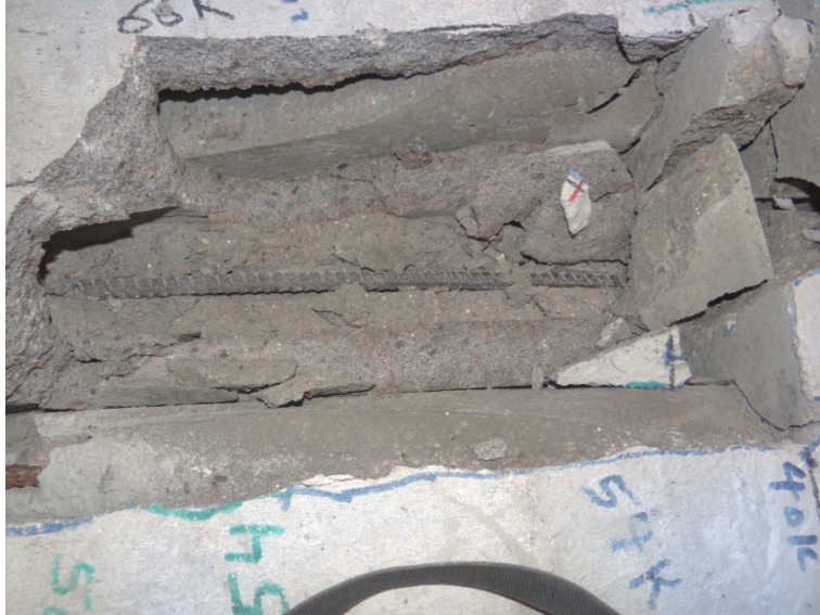
Figure 4-15 Failure in the planks due to debonding between grout and steel rebars.
