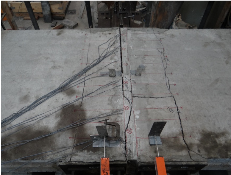
Figure 4-147 Cracks at the end of steel rebars in the hollow-core panel (north side).
