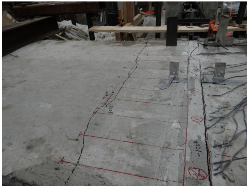
Figure 4-144 Separation between the plank (north side) and the connection; Crack at the end of steel rebars.
