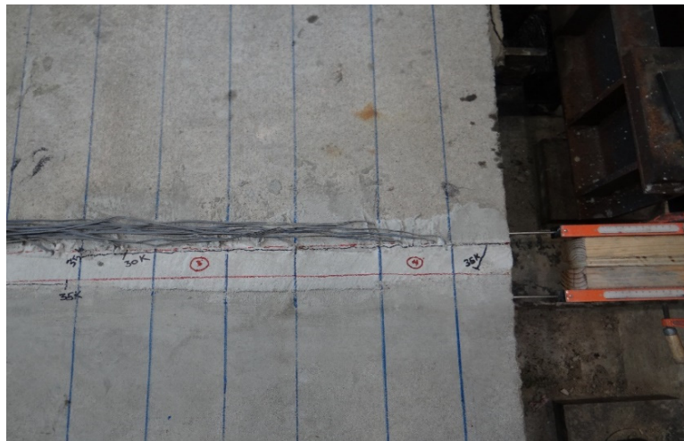
Figure 4-31 The developing and propagation of cracks at -35 Kips.
