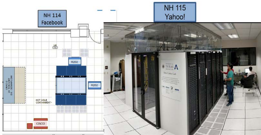
Figure 1-2: Data Center facilities at UTA
