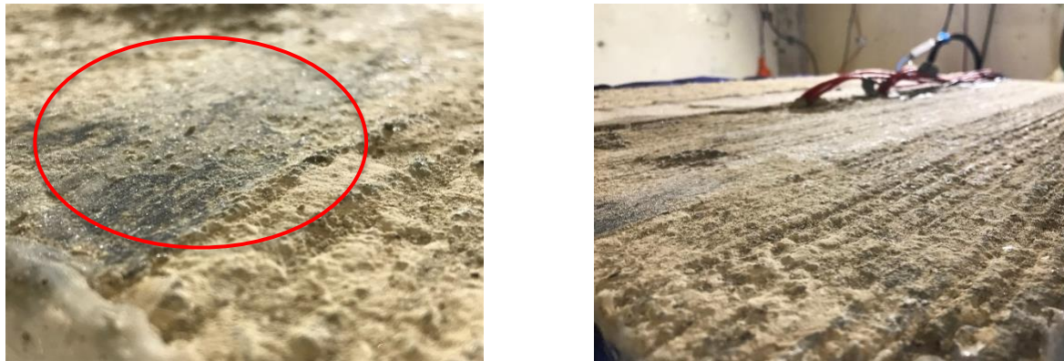
Figure 57. Light coating of frost on the surface of the slab
