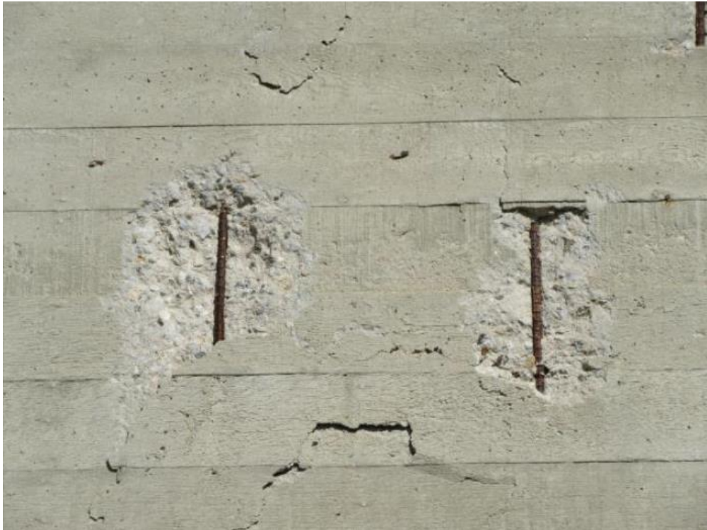
Figure 2.2. Delamination and spalling in a reinforced concrete wall (Harrer and Gaudette 2019).
