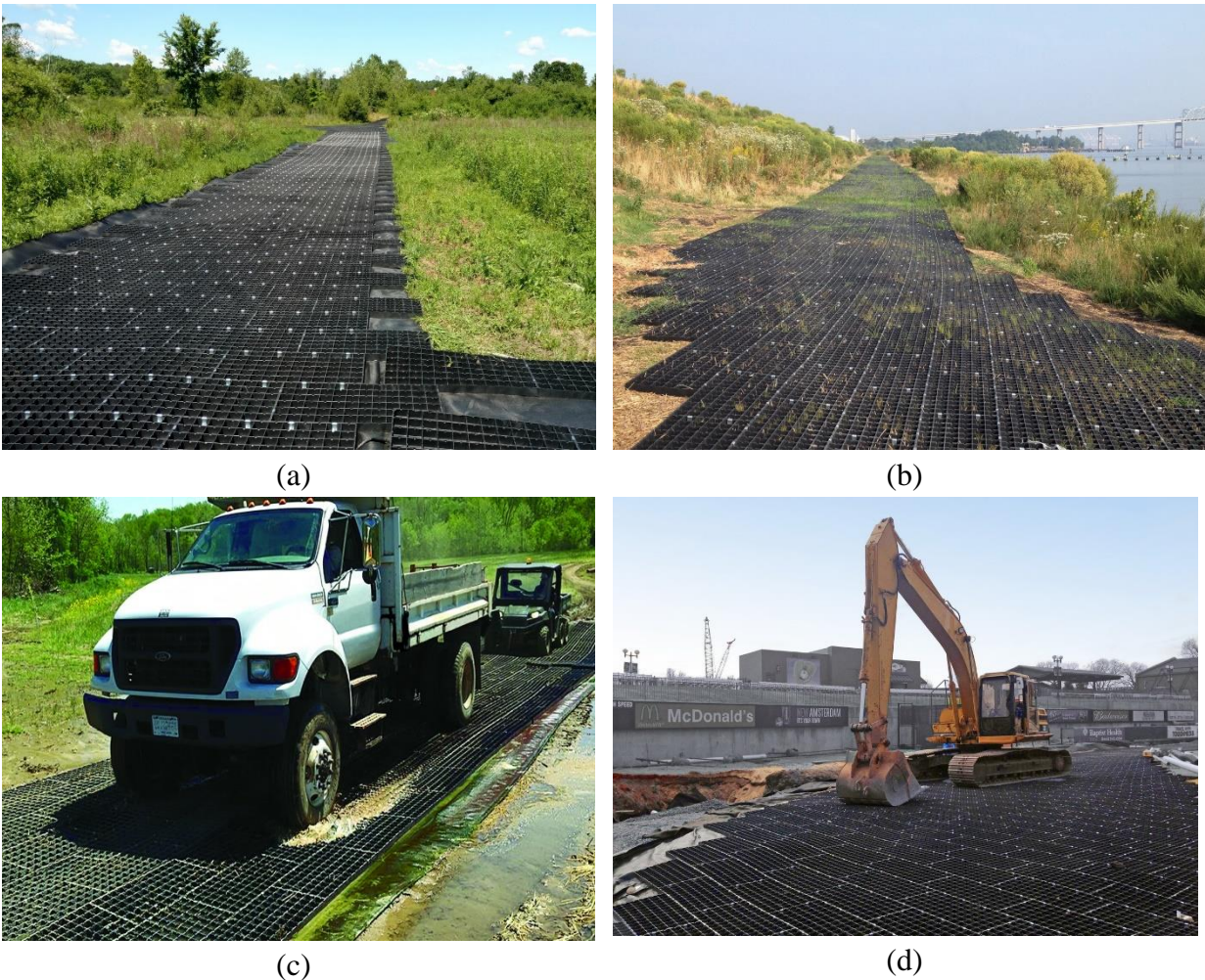
Figure 2.23: Different type's uses of construction mats. (a) site access over soft ground; (b) Minimal disturbance in environmental areas beside river; (c) heavy equipment access over wet ground (d) temporary site access and turf protection (Source: Presto Geosystems;
