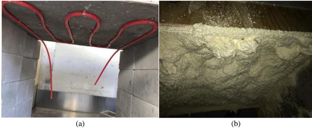
Figure 2.10. A lab experiment of the external heating system; (a) attached hydronic loops to the bottom of the concrete slab; (b) Applied spray foam to the bottom surface for thermal insulation (Hurley 2019)
