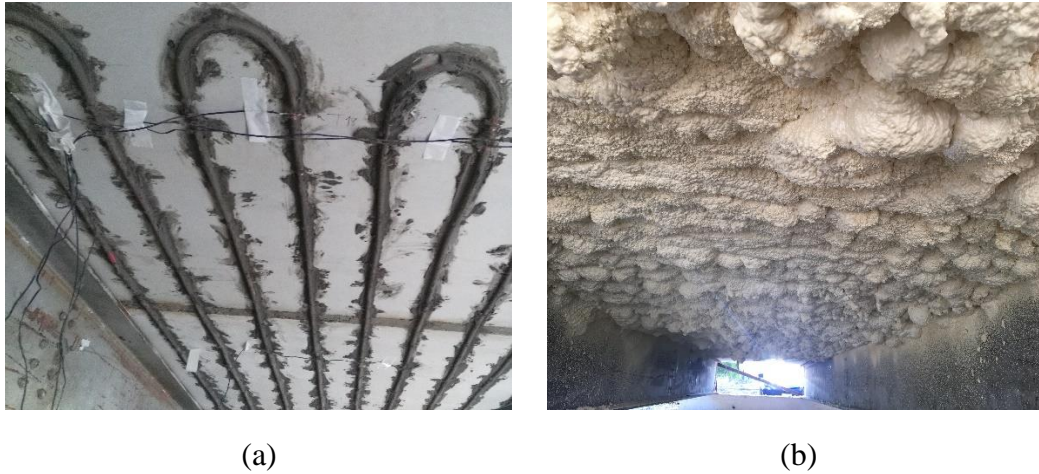
Figure 4.7. Installation of the hydronic loops: (a) Hydronic loops installed on the bottom surface of the externally heated zones, then covered by a cement paste, (b) A layer of polyurethane foam applied to the deck bottom
