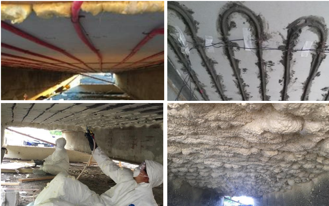
Figure 3.8. The construction process of stage 2: External hydronic loop and applying insulation foam.
