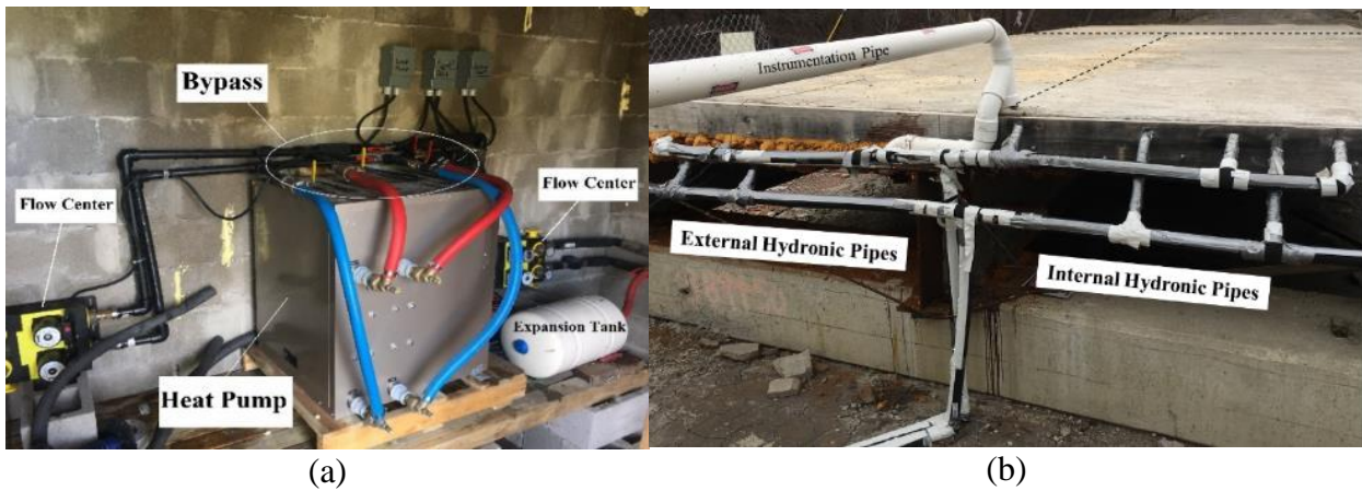
Figure 5.2. (a) Control room; (b) Bridge deck hydronic pipes
