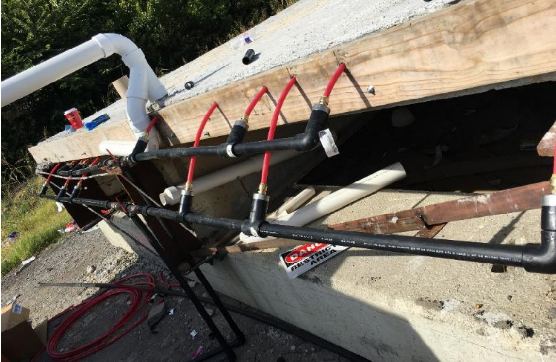
Figure 3.9. Hydronic loops inlet and outlet pipes
