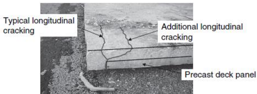
Figure 2-1: Longitudinal crack caused by shear (right crack) (Alvi et al. 2012)
