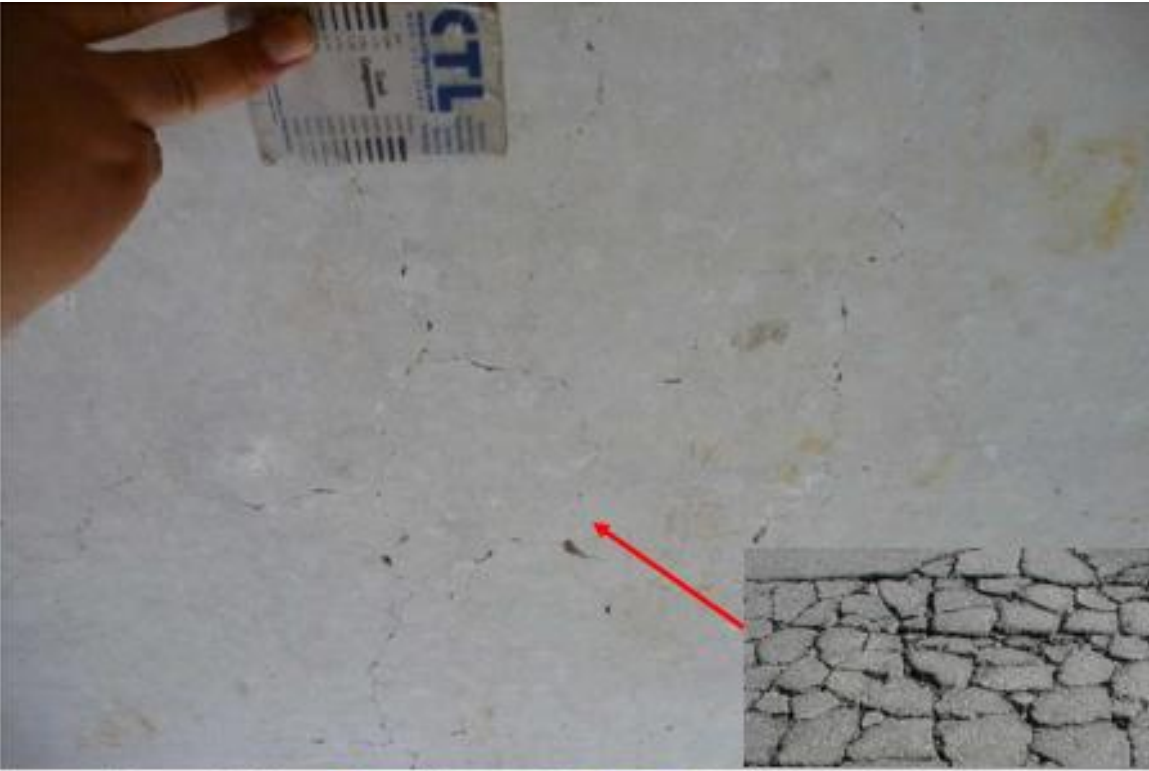
NOTE: Widespread hairline to minor alligator cracking (some with efflorescence) of Deck Panels between Girder Nos. 3 and 4 (from NW) in Span No 4. (This area is directly below patches in Deck surface.)
