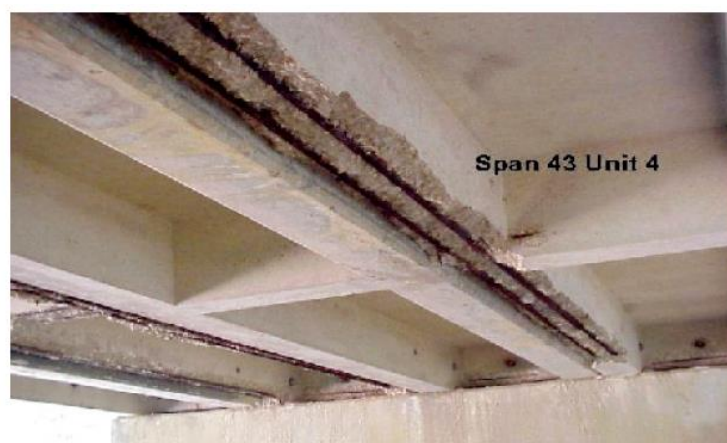
Figure 2-4: Deterioration of Jenkins' Ferry Bridge (Durham et al. 2004)
