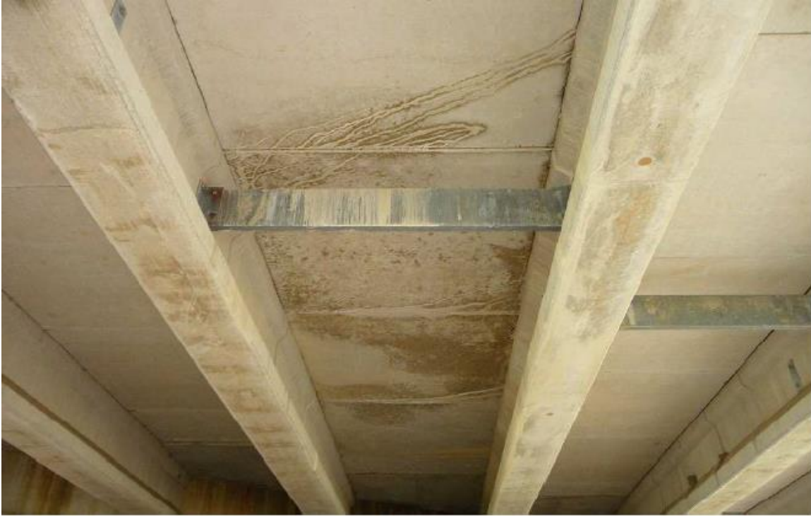
NOTE: Widespread hairline to minor alligator cracking (some with efflorescence) of Deck Panels between Girder Nos. 3 and 4 (from NW) in Span No 4. (This area is directly below patches in Deck surface.)
