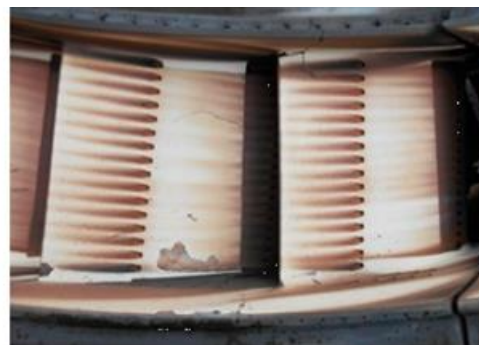
b) First-stage nozzles took a beating on this 7FA in cogeneration service.
