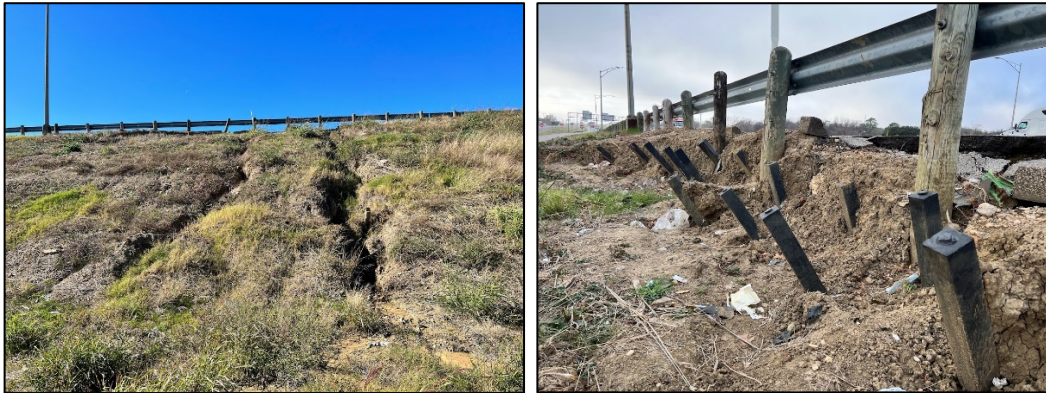
Figure 5.15 Surface Erosion in December 2021 exposing the RPP at the Crest.
