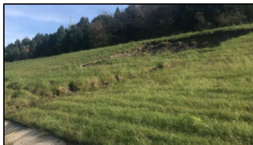
Figure 2.2 Shallow Slope Failure (Rauss, 2019).
