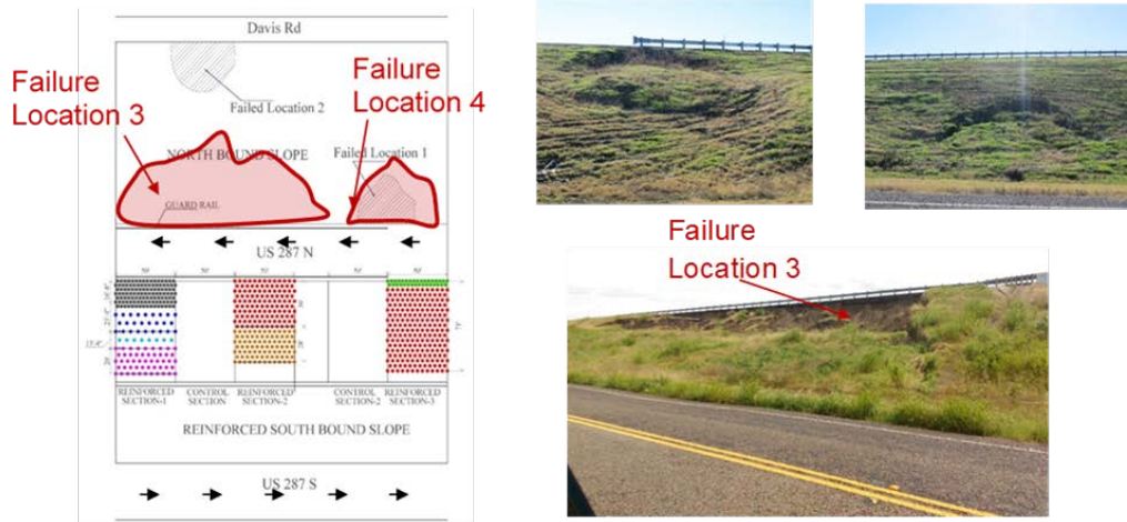
Figure 2.36 Slope failures observed in Northbound Control Slope (Khan, 2017)
