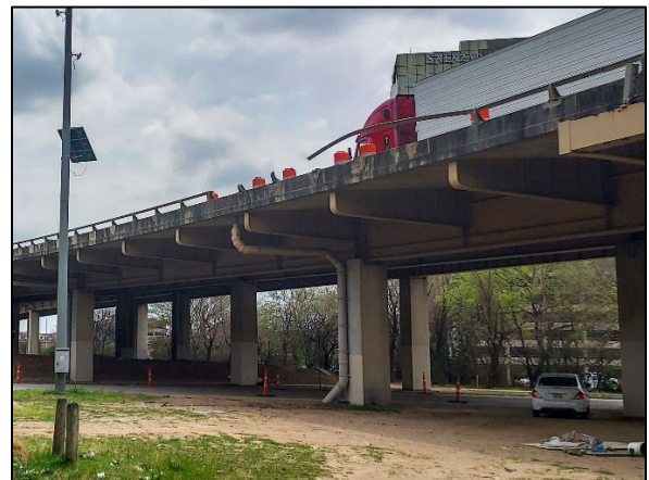
Figure 31 – Damaged Railing on I-345
