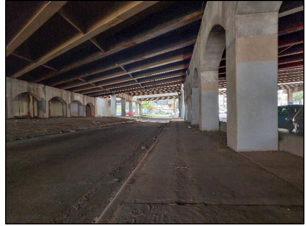
Figure 29 – Unsafe Conditions Under I-345 at Ross Ave
