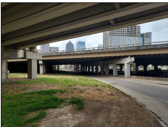
Figure 28 – Lack of Lighting Under I-345 at Ross Ave
