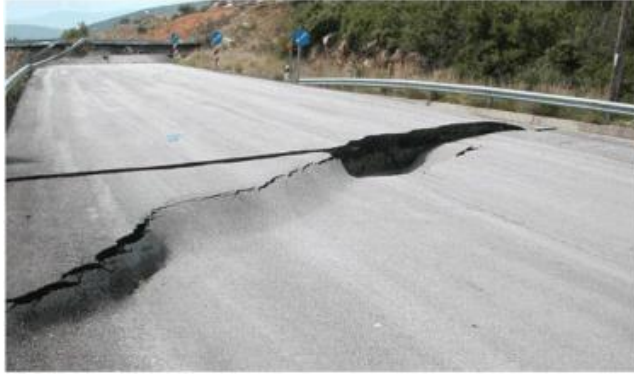
Figure 2-3 Road pavement defect duo to poor subgrade (U.S. Department of Transport).
