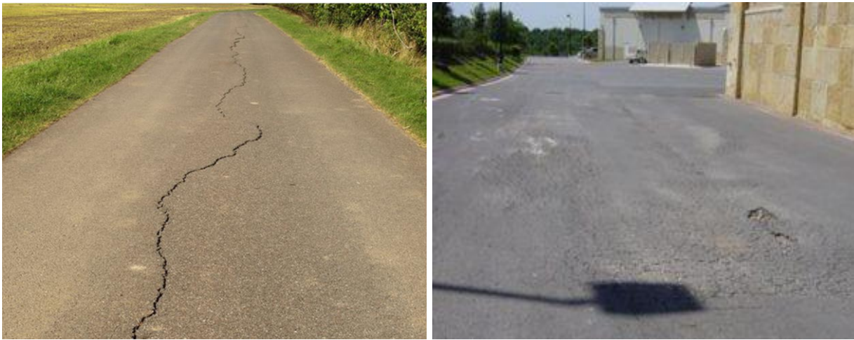
Figure 1-1 Premature failure caused by poor subgrade (roadwurx.com)
