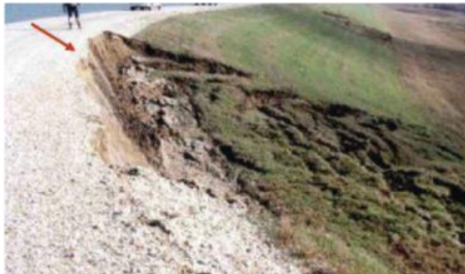
Figure 2-5 Slope failure of embankment caused by expansive soil (Jalal et al., 2020).
