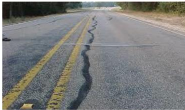
Figure 2-4 Typical longitudinal crack developed on pavements over expansive clays (Zornberg and Gupta, 2015).
