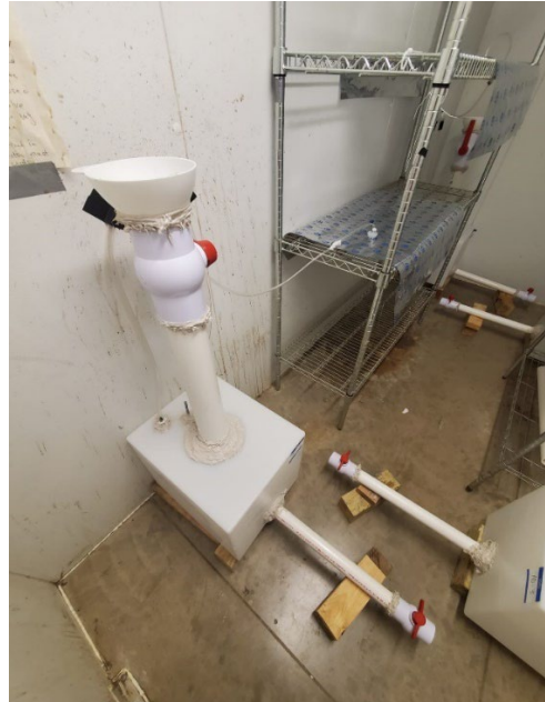
(b) Anaerobic Digester 2
