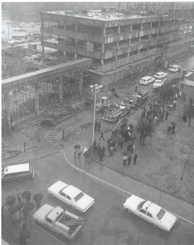
7.11 One of the few construction accidents at UTA occurred in 1970 when, during the construction of University Hall, the freshly-laid concrete roof of the theater collapsed. While the incident attracted much attention, there were no serious injuries.
