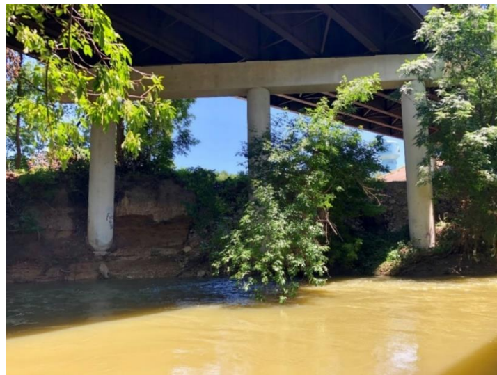
Figure 28: Existing Channel condition that has been eroded and scoured
