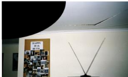
Figure 1.1 Exposed cracks in a residential building founded on expansive soil (Li et al., 2014)
