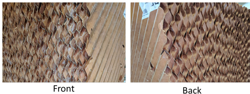
Figure 6: Scale deposition more pronounced at the inlet of the media pad
