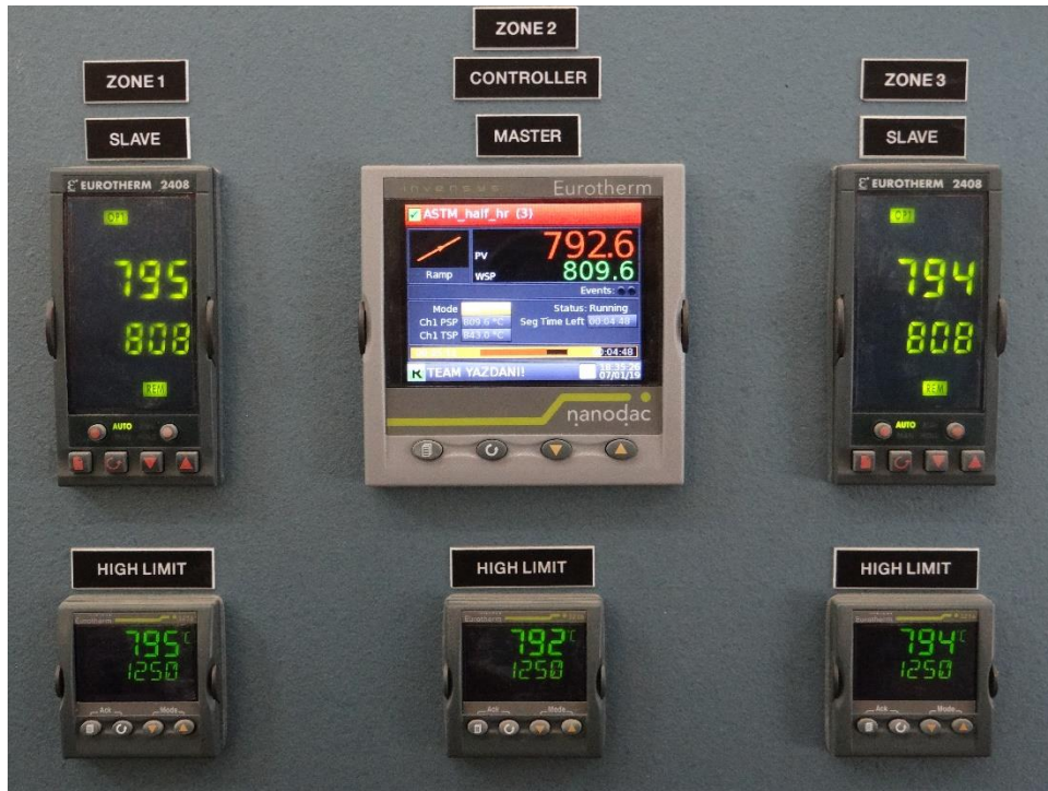
Figure 3.111 Controller of the furnace
