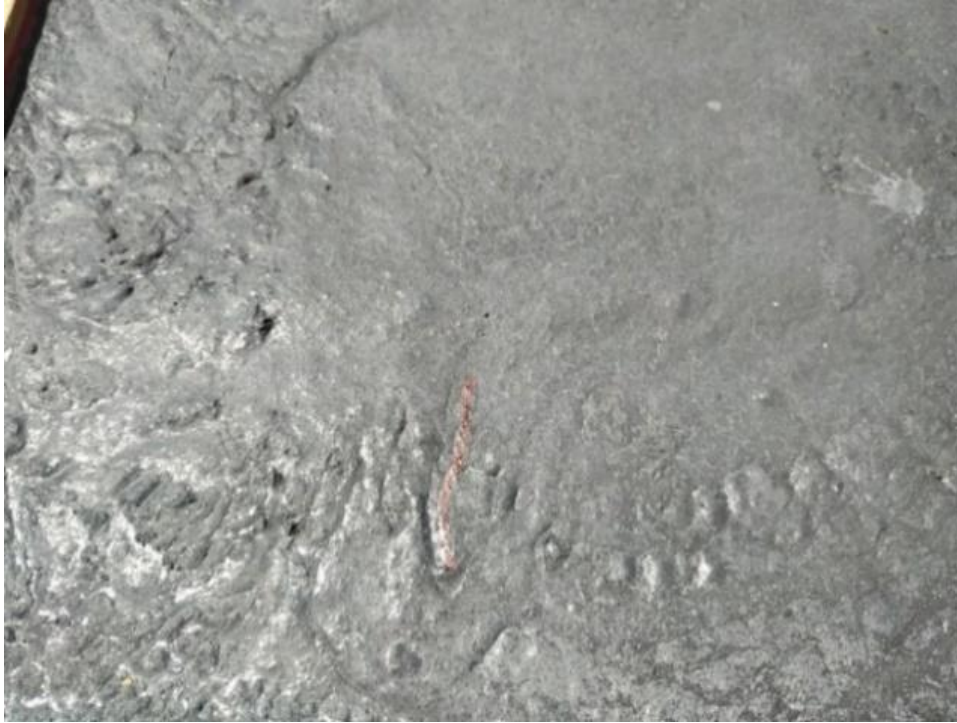
Figure 3.102 Small Cracks at UHP-FRC with No Curing
