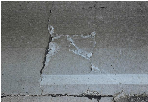
Figure 2-10. A typical CRCP punch-out distress
