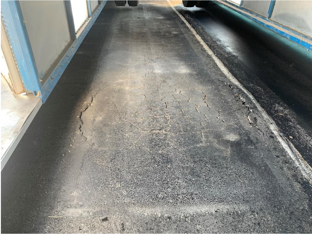
Figure 3.80 Surface cracking on section O after 350,000 passes
