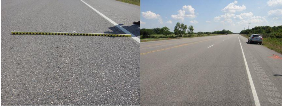
Figure 2.20 Excellent condition of RAP/ RAS test sections on SH146, Houston (Zhou et al. (2013)).
