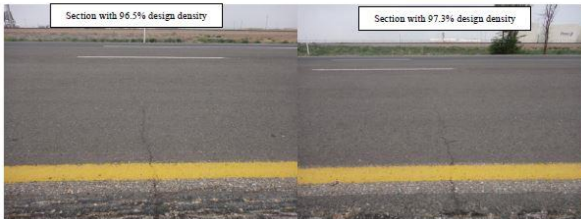
Figure 2.21 Reflective cracking of RAS test sections on US87, Amarillo (Zhou et al. (2013)).
