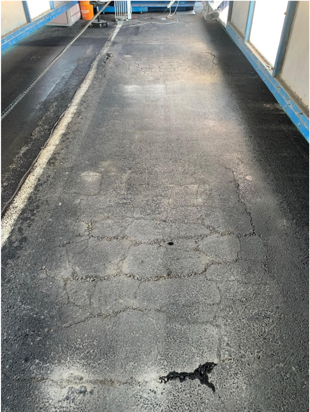
Figure 3.79 Surface cracking on section M after 300,000 passes
