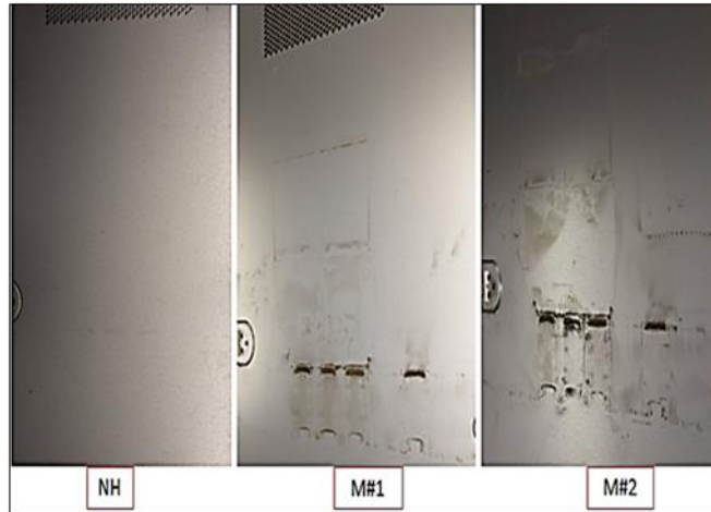
Figure 5-12: A comparison of dust deposition on the server chassis cover in (left) a clean laboratory data center (middle and right) in a modular data center located in polluted geography using an Indirect/Direct Airside economization unit [47]
