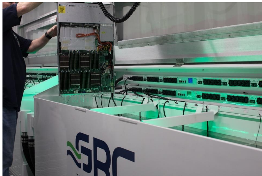
Figure 1-2 : Implementation of single-phase immersion cooling showing hot-swapping of server from dielectric fluid pool [12]
