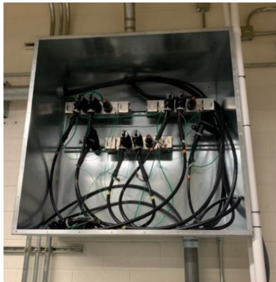
Figure 1.7: Photograph of the 4160 VAC distribution box installed in the laboratory.
