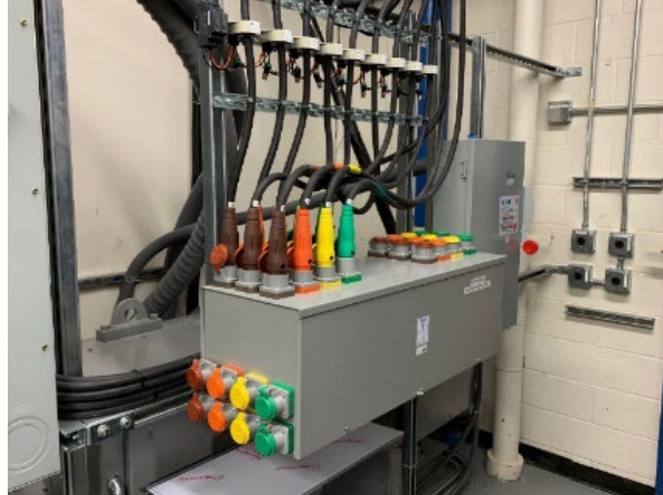
Figure 1.5: M-G or utility grid power distribution box.
