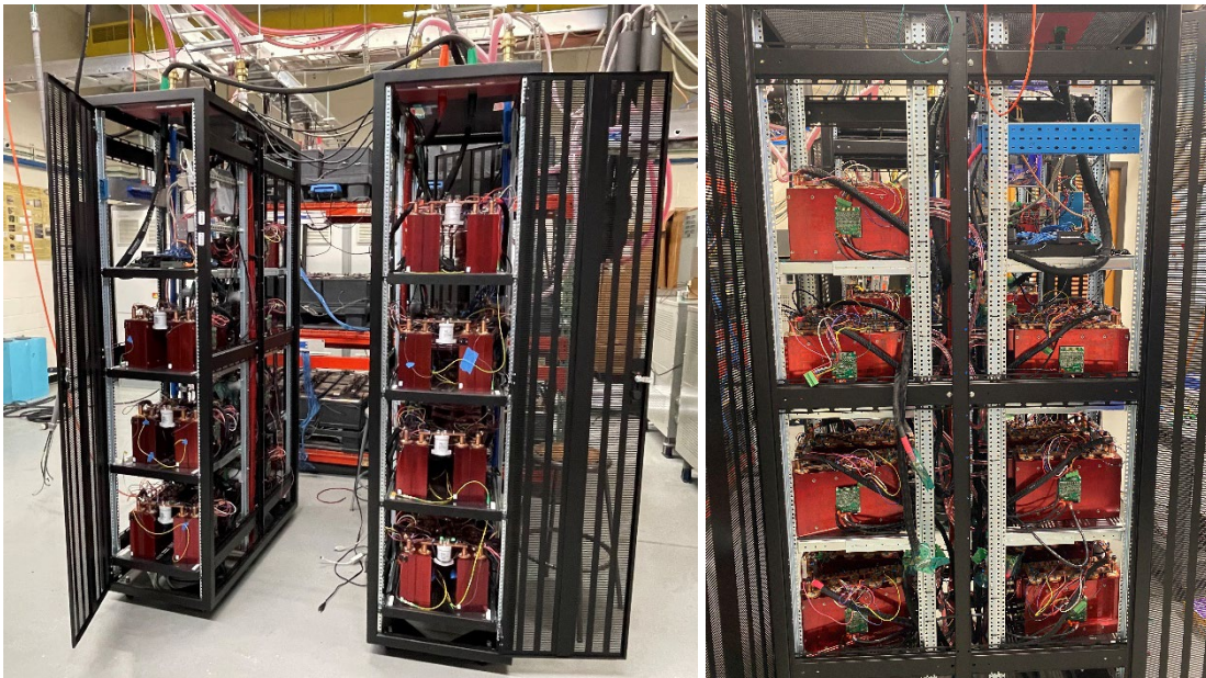
Figure 1.12: Photograph of the \sim 1 kVDC LFP-LI battery.
