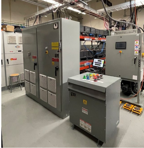
Figure 1.14: Photo of the Unico 150 kW, 480 VAC \leftrightarrow 1.1 kVDC bi-directional power converter (seen at left in photo) and isolation transformer (seen at lower right in photo).
