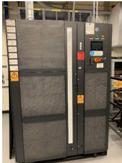
Figure 1.6: Photograph of the GE MV6000 power electronic drive.
