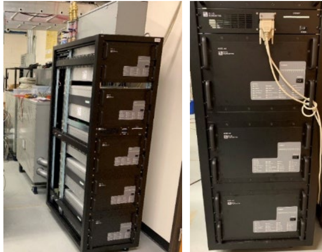
Figure 1.11: Photograph showing the installation of the three – 50 kW TDK Lambda power supplies used to convert 480 VAC to 1.2 kVDC (upper two supplies are the two 12 kVDC supplies and the lower three are the 1.2 kVDC supplies)
