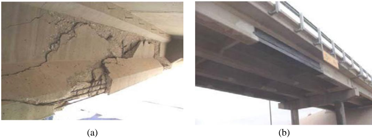
Figure 2- 27 Bridge Condition: (a) impact damaged; (b) impact damaged repaired with CFRP (Yang et al. 2011)
