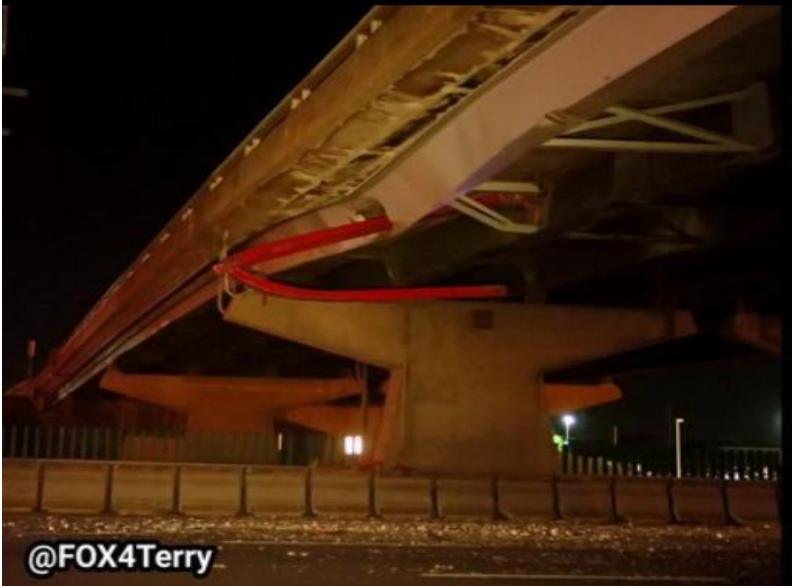
Figure 1- 5 Wrecker punched through the steel beam (Fox 4 News 2017)
