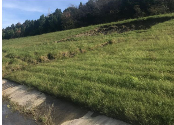
Figure 2-11 Shallow slope failure near eastbound IH20 in Dallas, Texas (Rauss,2019).
