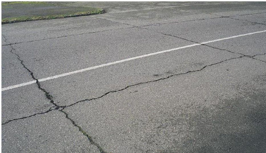
Figure 2.11. Low Temperature Cracking (Ahmad and Khawaja, 2018)
