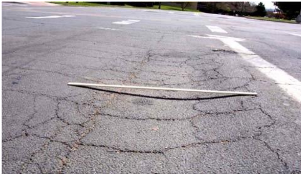
Figure 2.9. Rutting of pavement (Sarah et al 2017)
