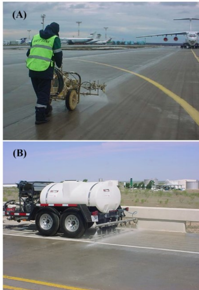
Figure 2.13 Application of the DCE solution by spraying onto cured concrete for an airport runway (A) and a pavement (B) (Al-Jabari 2022)
