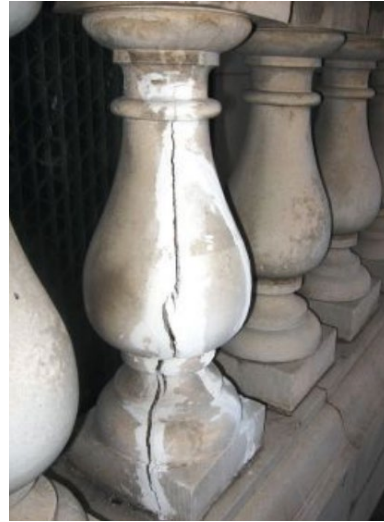
Figure 3.8 Cracked baluster (Lucy)
