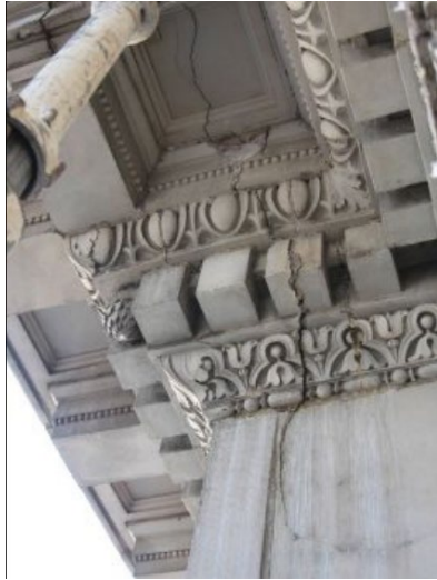
Figure 3.7 Cracking in overhead terra-cotta units (Lucy)
