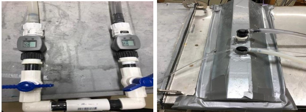
Figure 2-6 shows Digital water flow meter on each water supply and Separate water distribution headers
