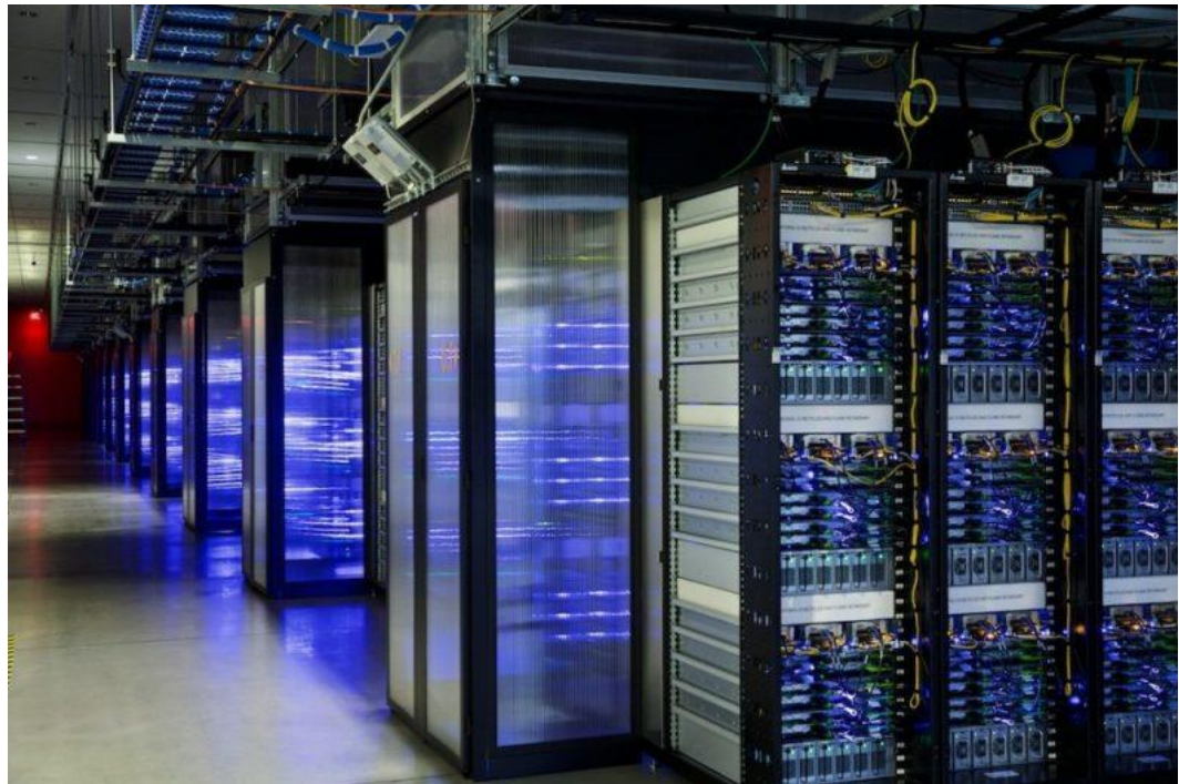
Figure 1-1 Facebook Data Center [9]
